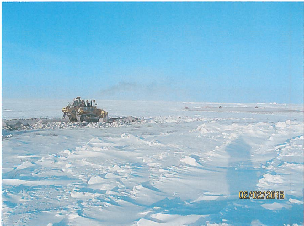
Figure 4. Construction of a road to the “Temporary North Laydown Area”. Once completed, the road will alleviate traffic congestion/conflicts between mining trucks and winter road traffic bringing in equipment & materials. The pad in question is temporary in nature, and will eventually become the mines Course PK Pile once temporary storage needs are over (i.e., September, 2016).
