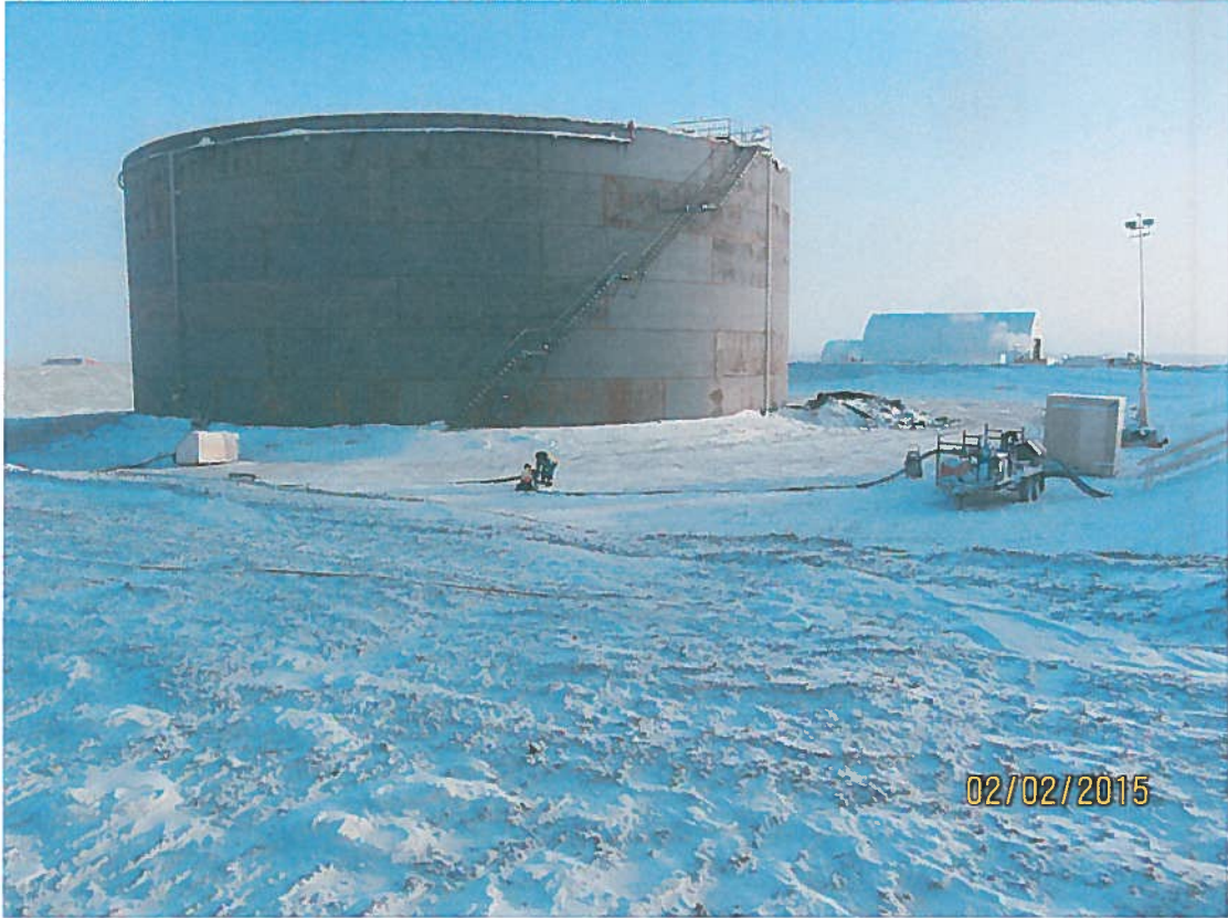
Figure 1. Work on the transfer of fuel to the 18 Million L Tank Farm.
