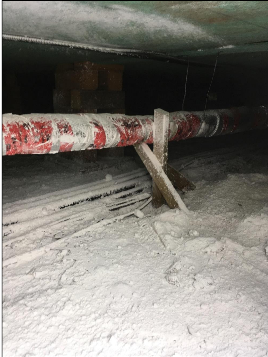
Photo showing the replaced pipe after corrective actions were completed. Blocking was added as extra support beneath the metal hanger supported sections of the pipe.
