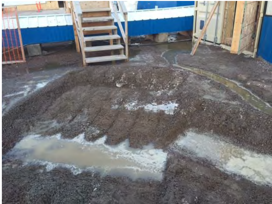
b. Sump to collect/contain spread of overflow excavated outside of Emergency Overflow Lift Station.
