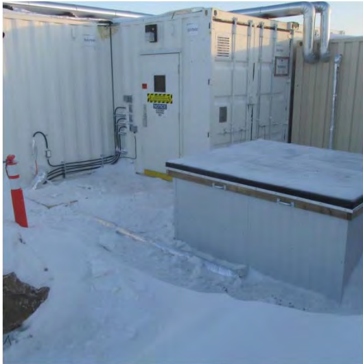
Nov. 16, 2014 – STP showing winterized pipe
