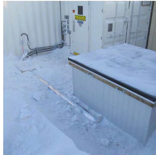
Nov. 16, 2014 – Winterized pipe and exterior tank
