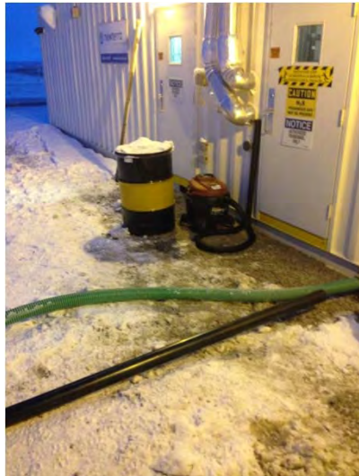
Oct. 16, 2014 – Photo of spill outside STP showing frozen pipe
