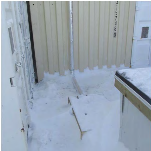
Nov. 16, 2014 – Winterized pipe and exterior tank
