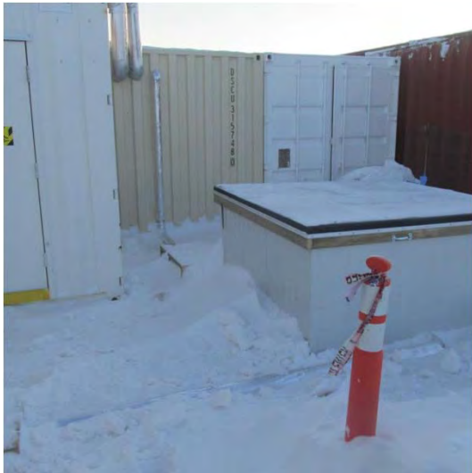
Nov. 16, 2014 – Winterized pipe and exterior tank
