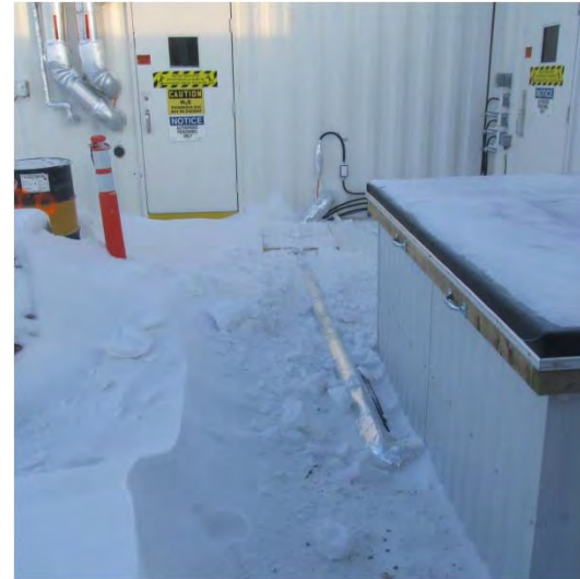
Nov. 16, 2014 – Winterized pipe and exterior tank
