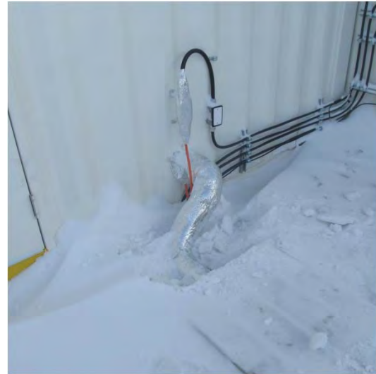
Nov. 16, 2014 – Winterized pipe and heat trace
