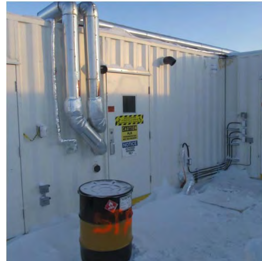
Nov. 16, 2014 – Winterized pipes
