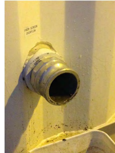
Oct. 16, 2014 – Exterior hose connection
