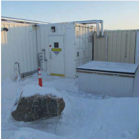
Nov. 16, 2014 – Winterized pipe and exterior tank
