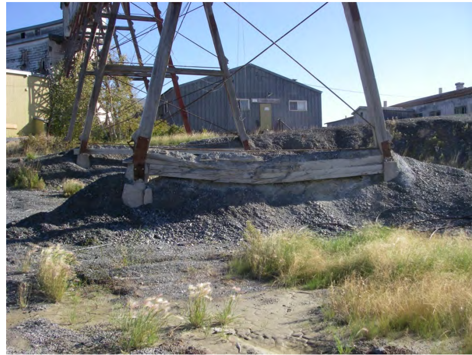
September 2011 – Damaged support frame and concrete support pier
