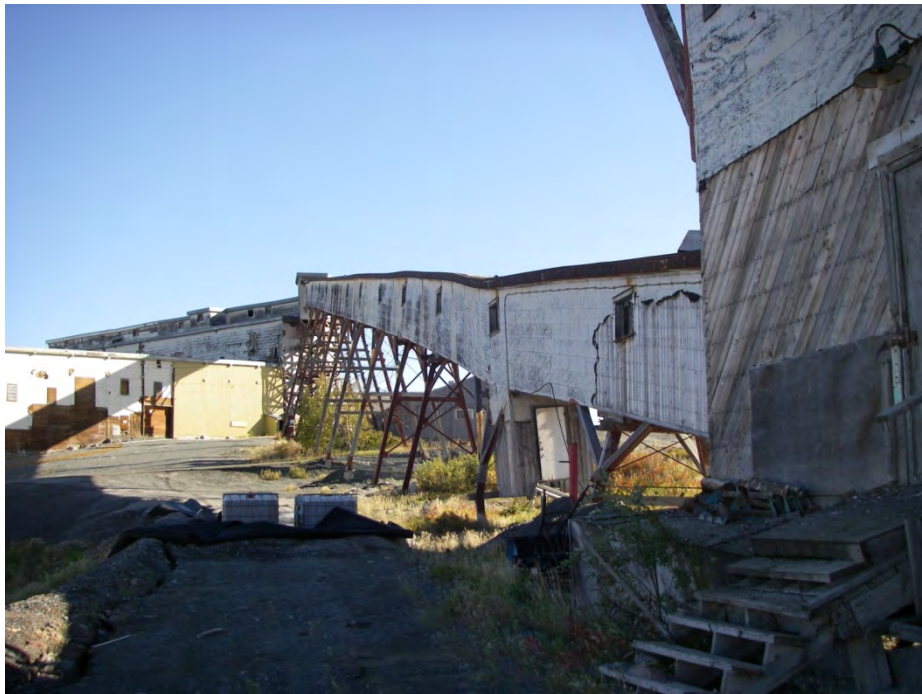
September 2011 – Uneven roof line indicates structure is moving
