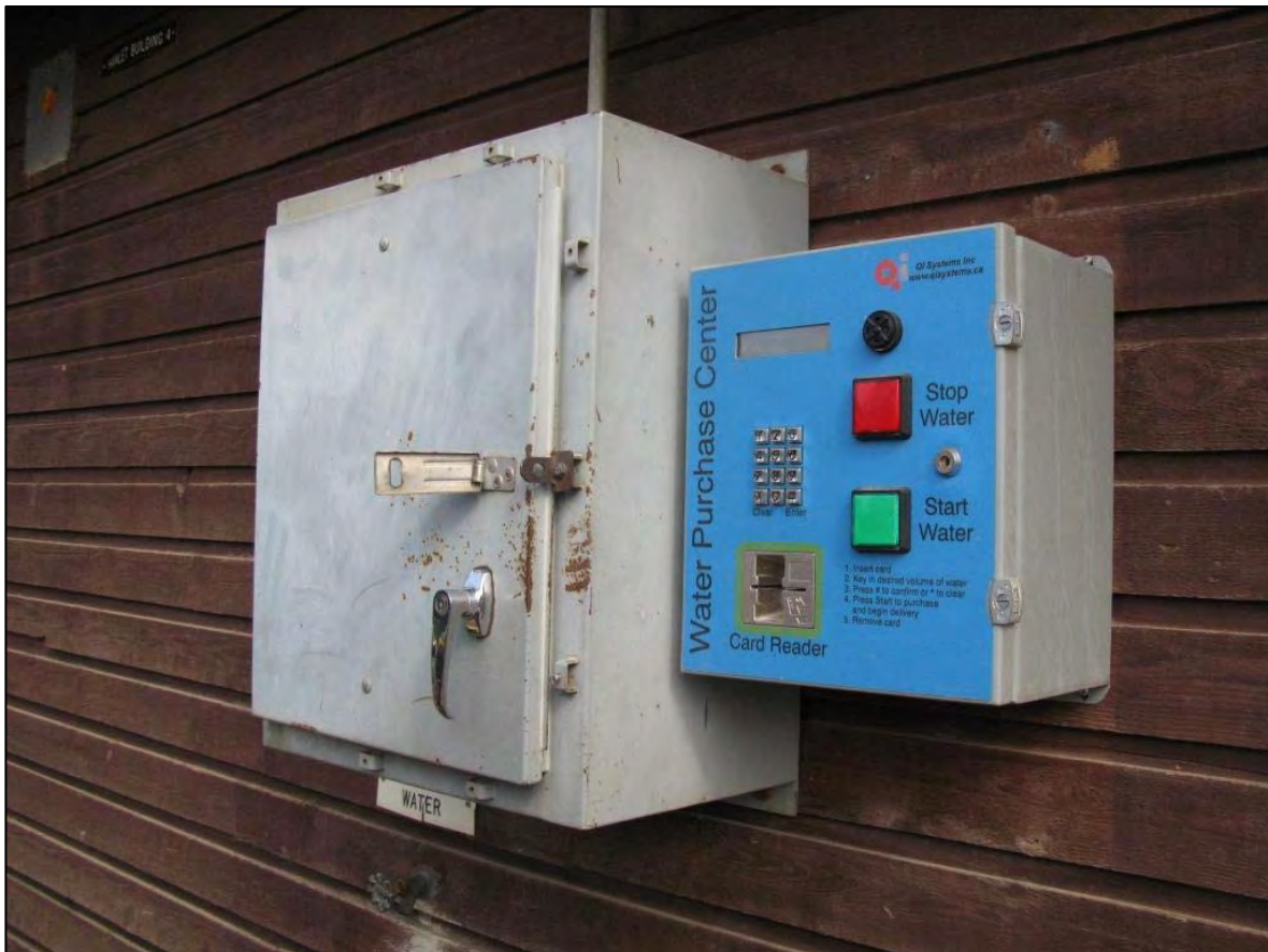
Figure 2 A new card lock reader has been installed as part of the water truck fill station at the water treatment plant.
