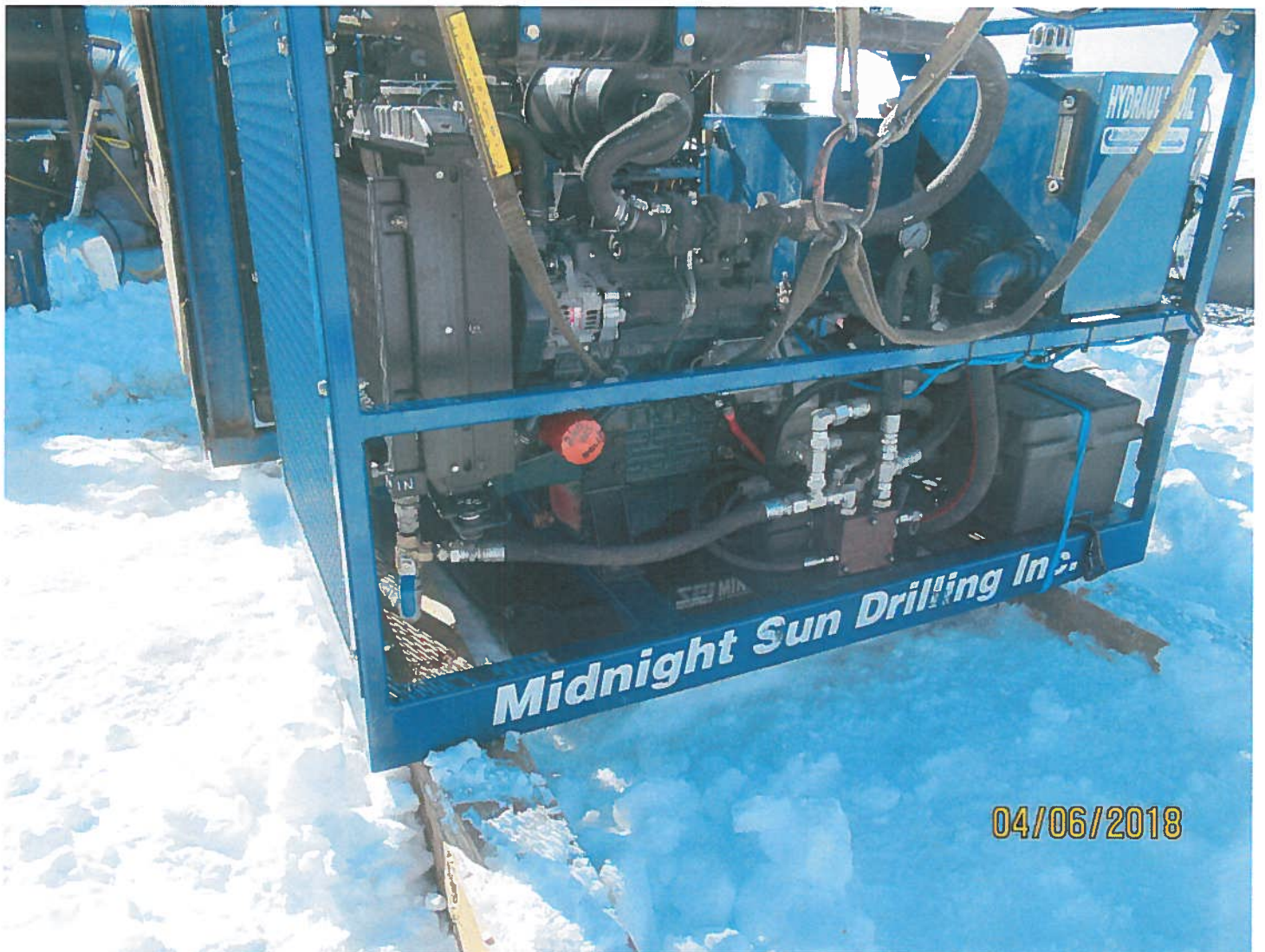
Photo #7 - MV2012C0009 - Dominion Diamond Mines ULC Generator appeared to be operating cleanly and secondary containment was present.
