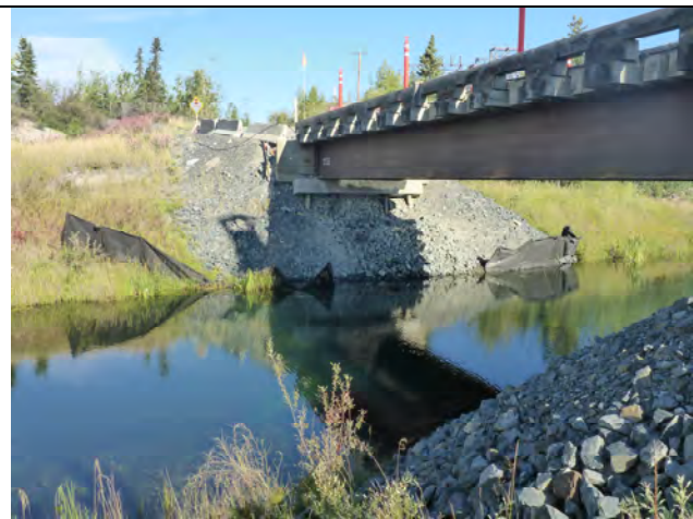
Photo 2: Northwest view from under the bridge towards the location of the spill.
