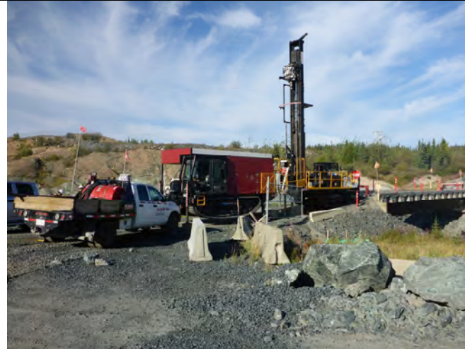
Photo 1: Overview of the final drilling location for the bridge stabilization project. (Looking west from the east side of the bridge)
