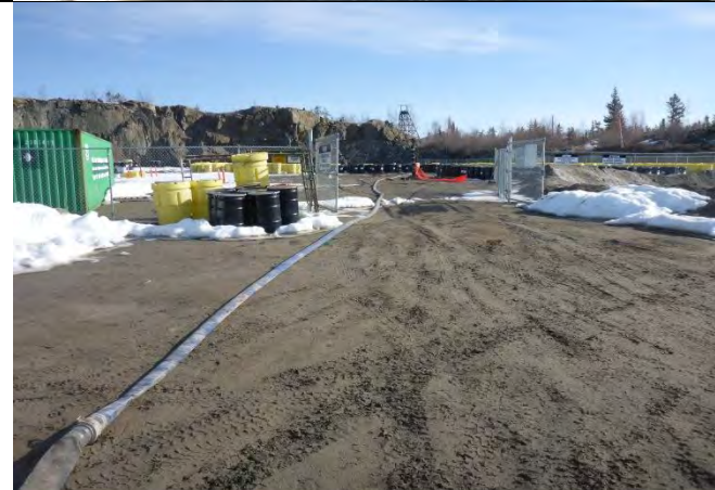
Photo 4: Piping to be used to pump the flooded area in Photo 3 to Northwest Pond.
