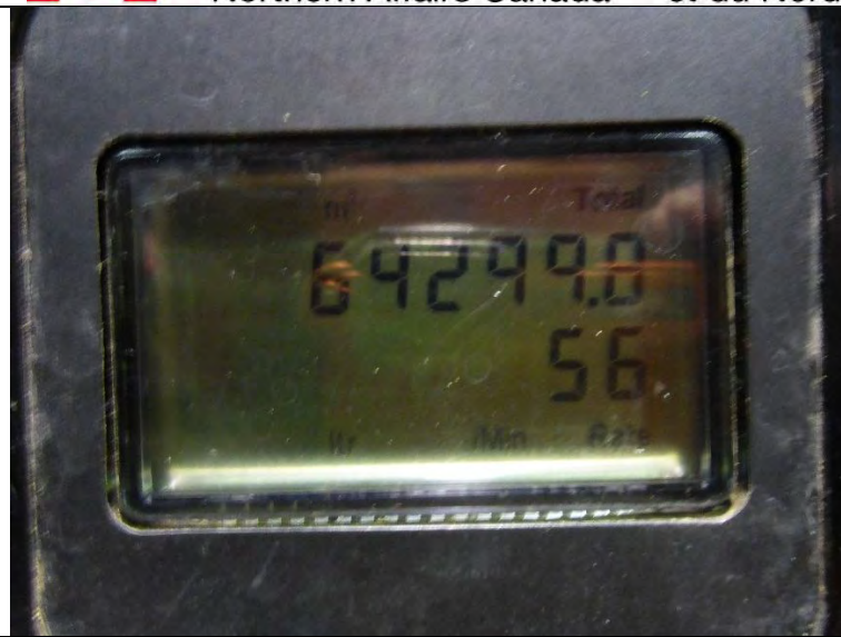
Photo #1: Close up of the water meter intake.
