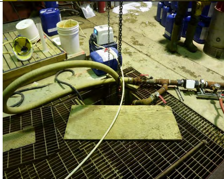
Photo #3: Chlorine being injected at the water treatment plant.
