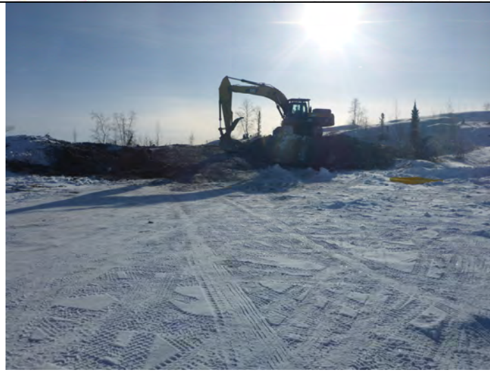
Photo #1: Overview of the excavation of material within 100 meters of the OHWM on Zenith Island.
