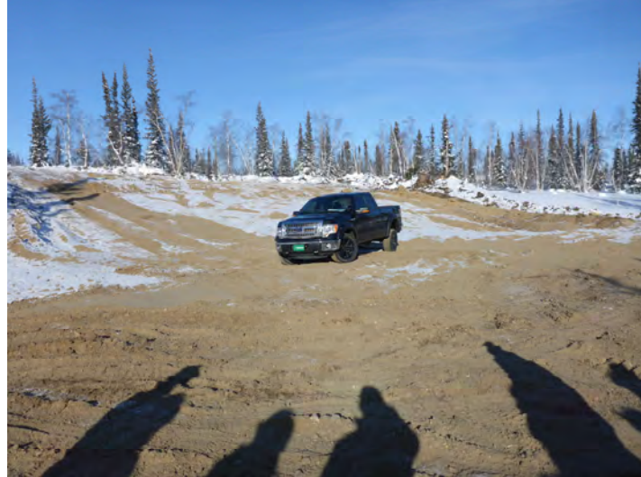
Photo #3: Overview of the tailings cover on Burnt Island. Note that this will need to be regraded to ensure that ponding does not occur.
