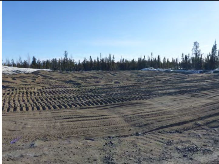
Photo #11: Excavated waste rock and contaminated soil area located at Kidney Pond.
