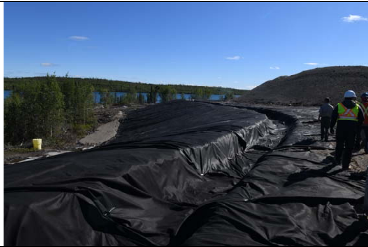
Photo #6: Overview of the geotextile liner placed over the diversion trench and down the slope of the cap to the toe drain.
