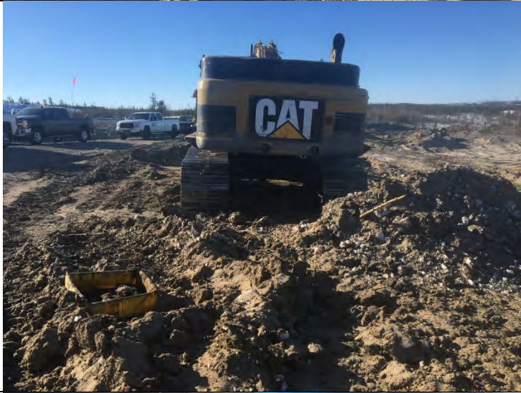
Photo #6: CAT with no Drip tray underneath.
