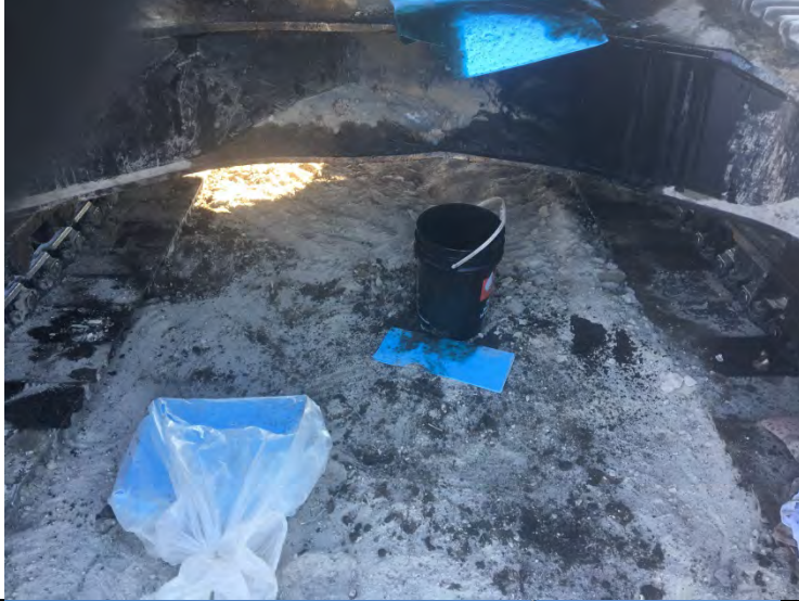
Photo #7: Spill of Hydraulic oil leaking on the ground and around the CAT at Westbay.
