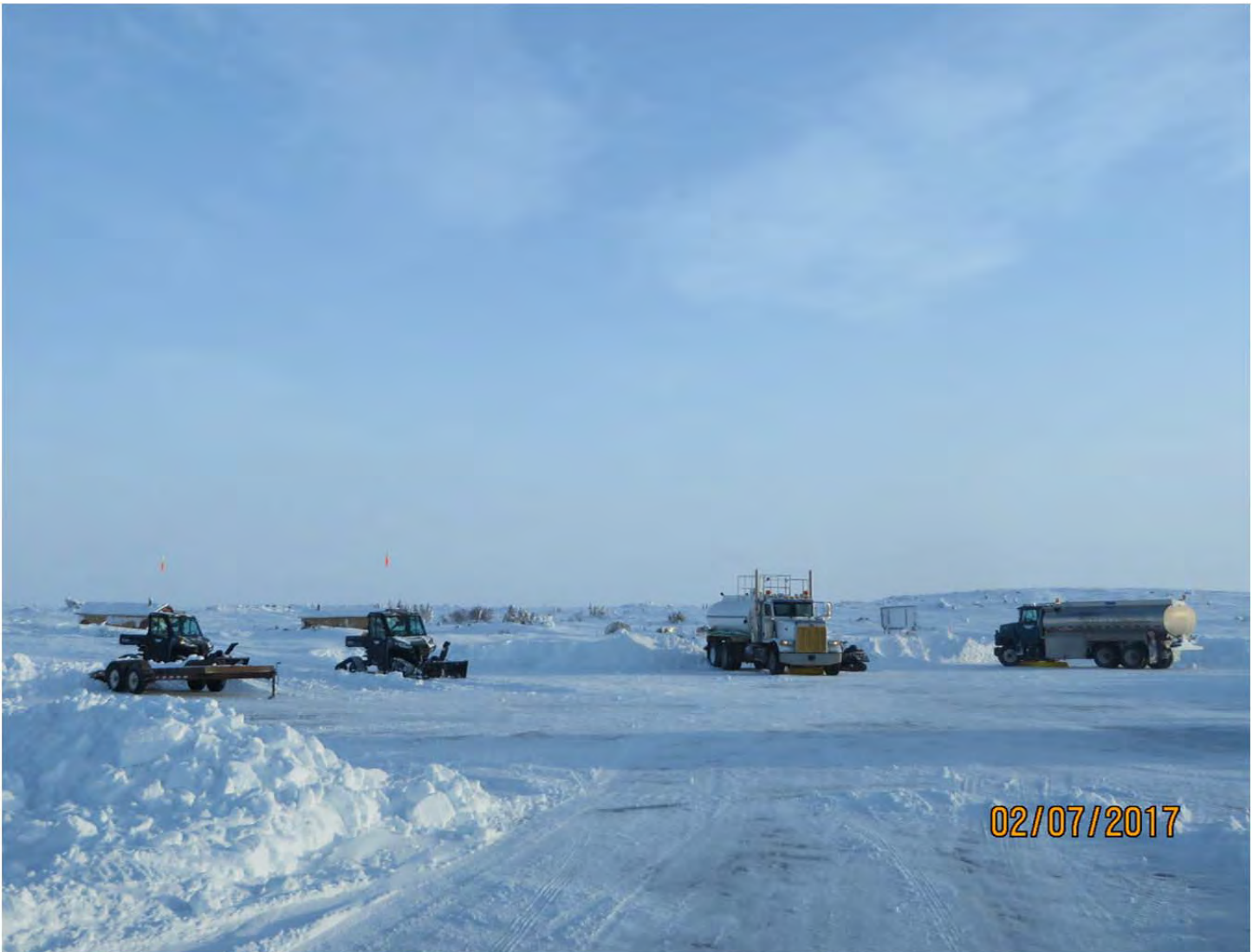
Photo #1 - MV2016X0011 - INAC-CARD - Tundra Equipment staged on the east side of Mackay Lake for the construction of the winter road to Tundra Mine.
