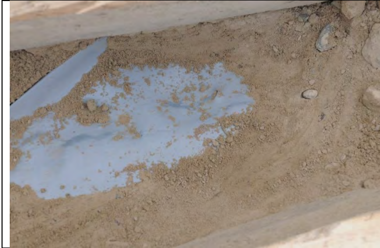
Photo #10: One of several holes found in the impermeable membrane during the inspection of the berm.
