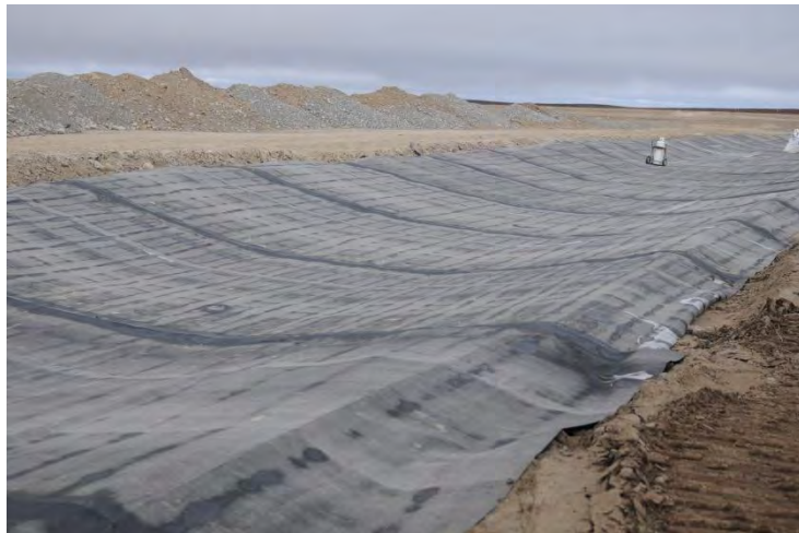
Photo #11: Liner being placed in the drainage channel connecting Mill Pond to Lower Pond.
