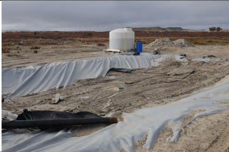
Photo #13: Wash berm which was used to rinse vehicles coming out of the tailings area has been ripped and no longer usable.
