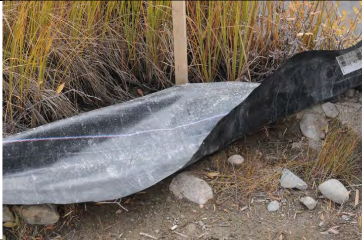
Photo #16: Silt fence around the bridge near the airstrip not installed properly. The top of the silt screen should be affixed to the posts to ensure it can't fold down.
