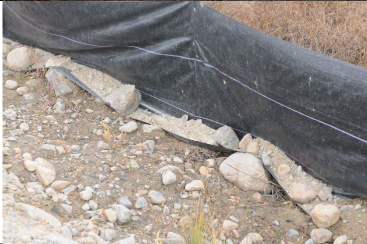
Photo #17: Improper installation of silt screen. The filter fabric dam should be appropriately embedded in the ditch bottom and sides (e.g. 100 mm minimum) to prevent the movement of fines under or around the dam.
