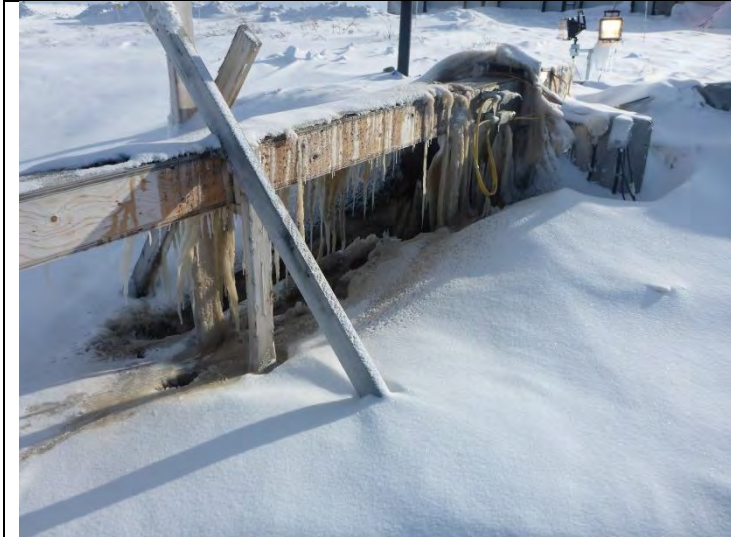
Photo #10: NT/NU Spill 18-061. Unauthorized sewage discharge from tank to lagoon.
