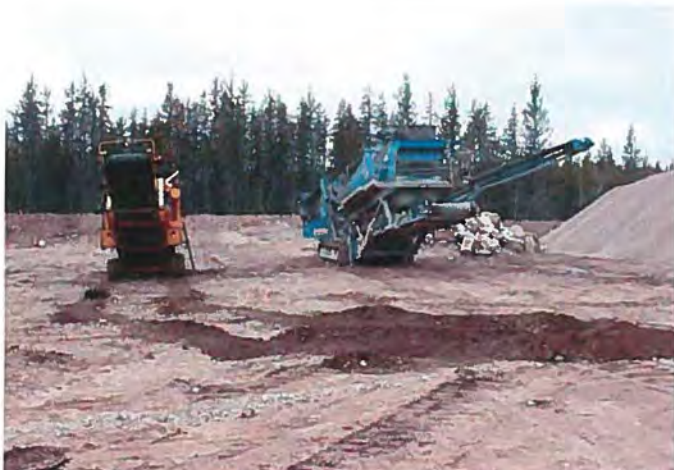
Site 2: Crushers not being used
