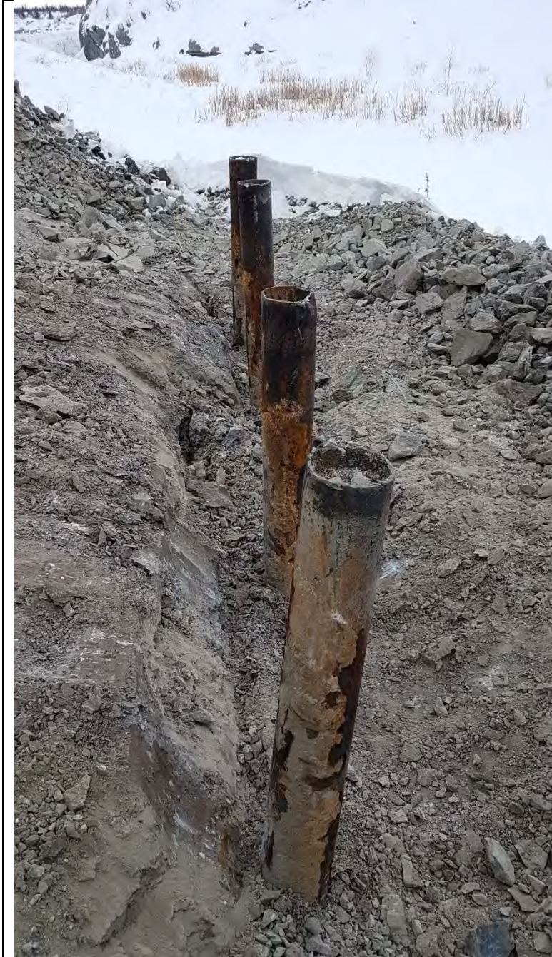
Photo #5: The older piles that will be replaced prior to the replacement of the bridge.
