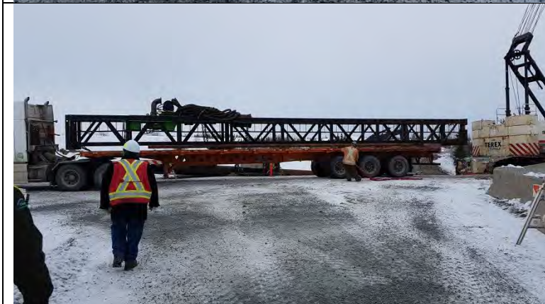
Photo #2: Overview of a load of material needed for the bridge repair.
