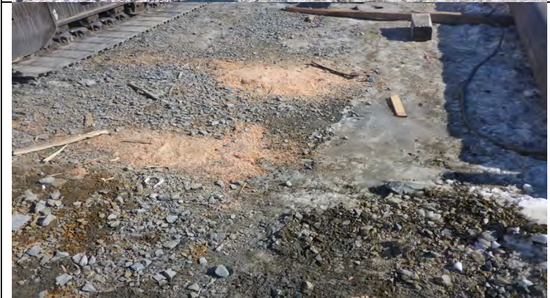
Photo #4: Area where approximately 1L of hydraulic oil spilled and was reported.
