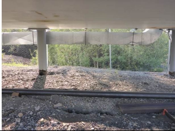
Photo #2: View of the ground under the building where spill #16-248 occurred. Note there is no sign of the spill reaching the surrounding environment.
