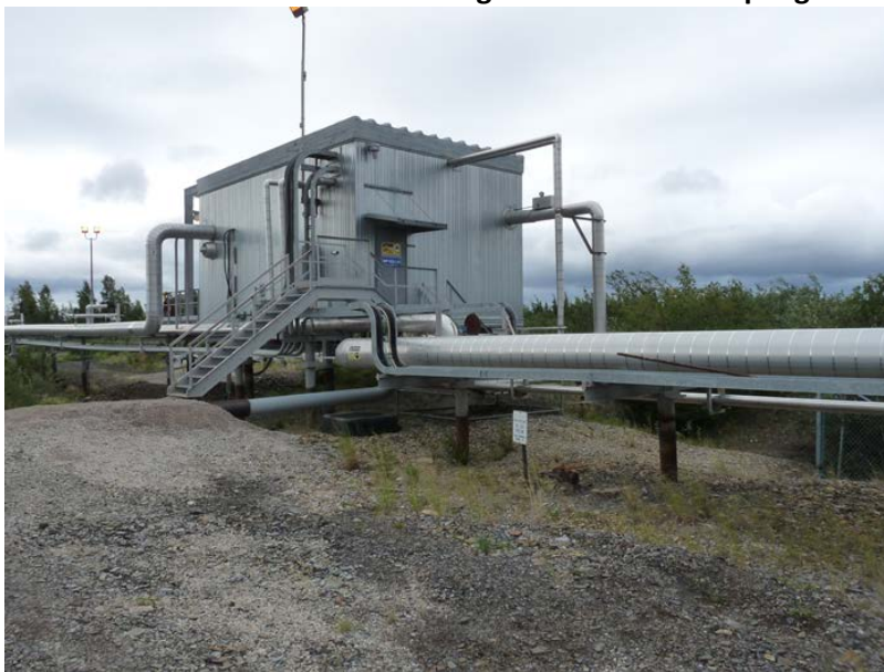
Photo A: Inlet Water Intake Building and S03L1-01 Sampling Location
