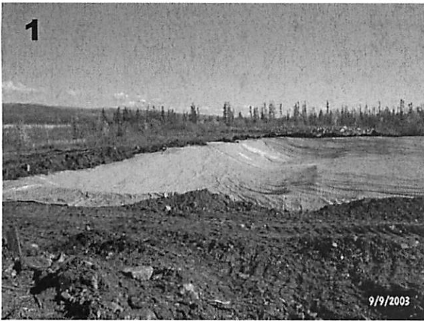
Geomembrane liner covers the base and perimeter berm of the LTU
