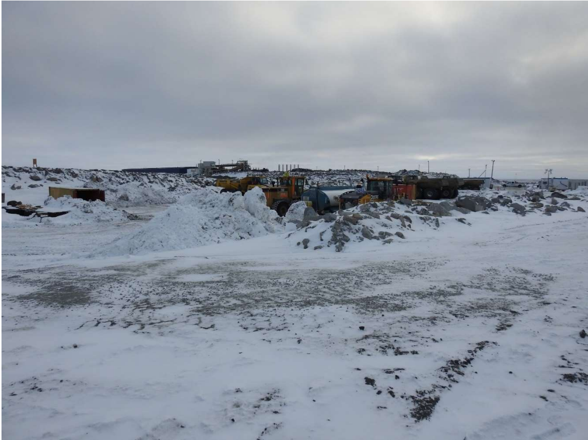
Figure 3 Spill 2020401 after scraping of area occurred and recovered FPK slurry taken to PKCF. Some frozen material remains to be recovered in spring 2021.
