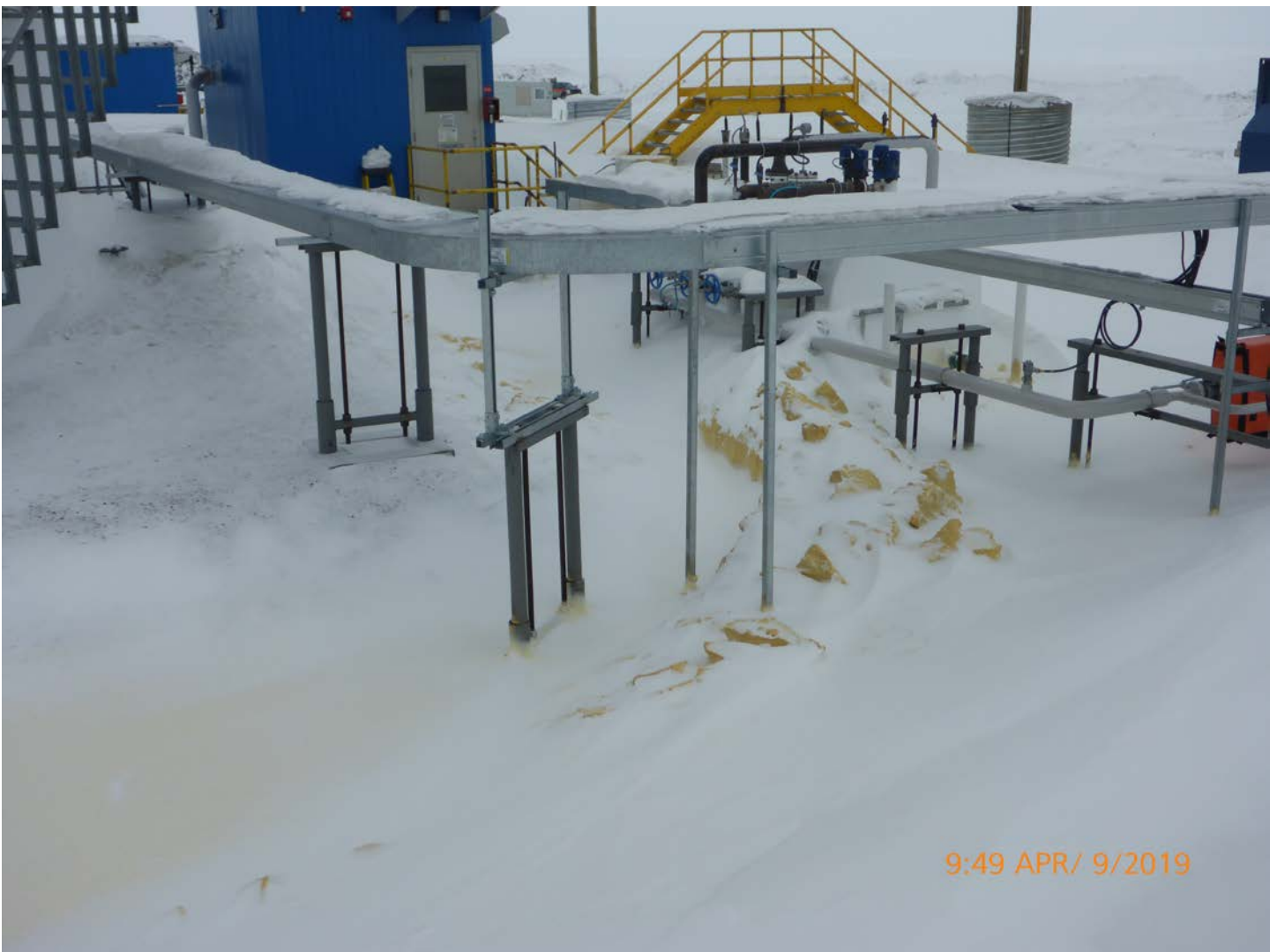
Photo 12 – Tank Farm Spill #2019127 – 100% of the diesel spilled was within lined containment and the containment berm worked as designed. There was no evidence of seepage from the berm at the time of inspection.
