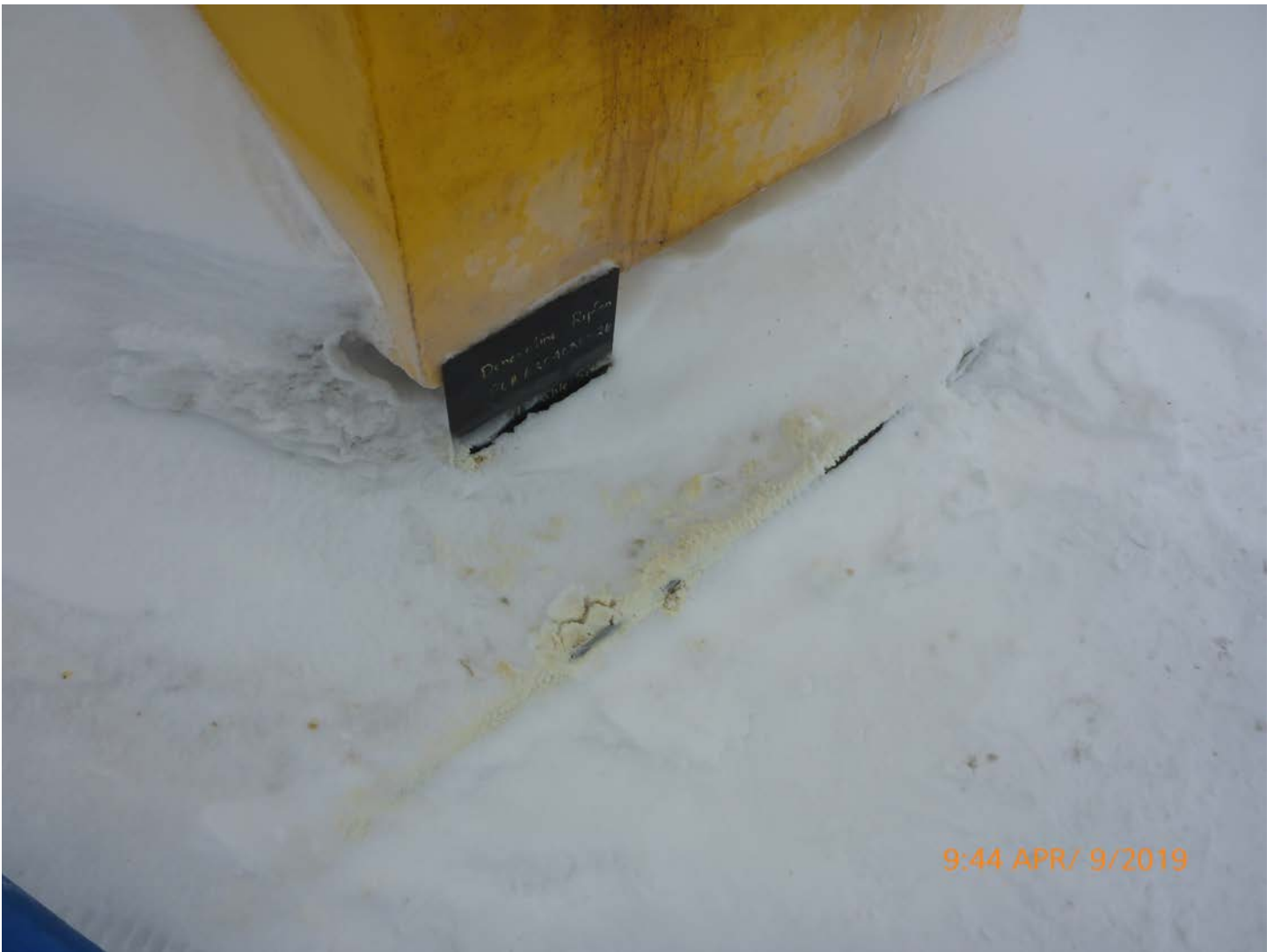
Photo 7 – Sable Refueling Station – Some minor spillage was identified within the containment tray at the refueling station.
