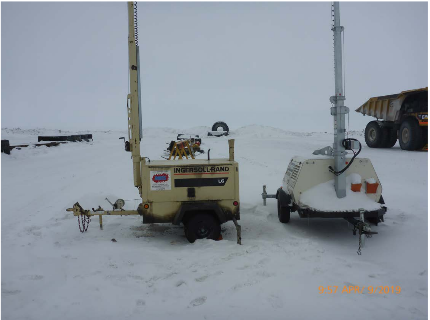
Photo 3 – Sable Laydown – Light plants are staged in the sable laydown. These light plants are equipped with integrated drip trays that satisfy Condition 37 of the Permit.
