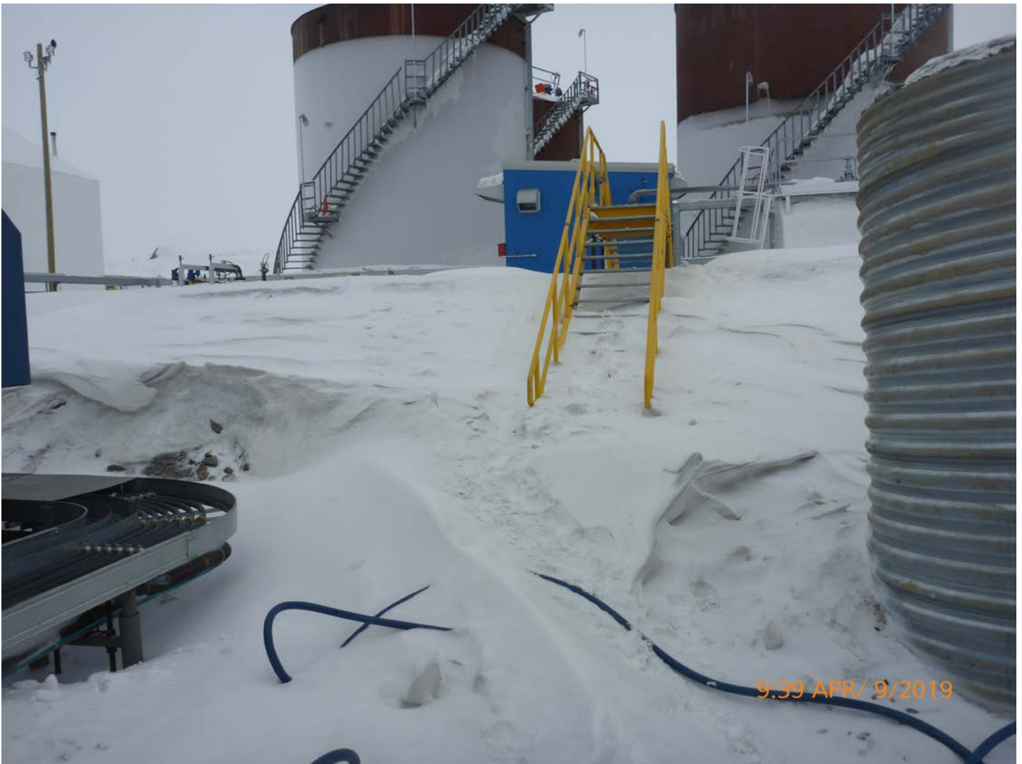
Photo 11 – Tank Farm Spill #2019127 – Access to the day tank in the sable fuel farm was snowed in which made the tank difficult to inspect. The Inspector recommends better maintenance at the access points to the tank farm containment to facilitate inspections.
