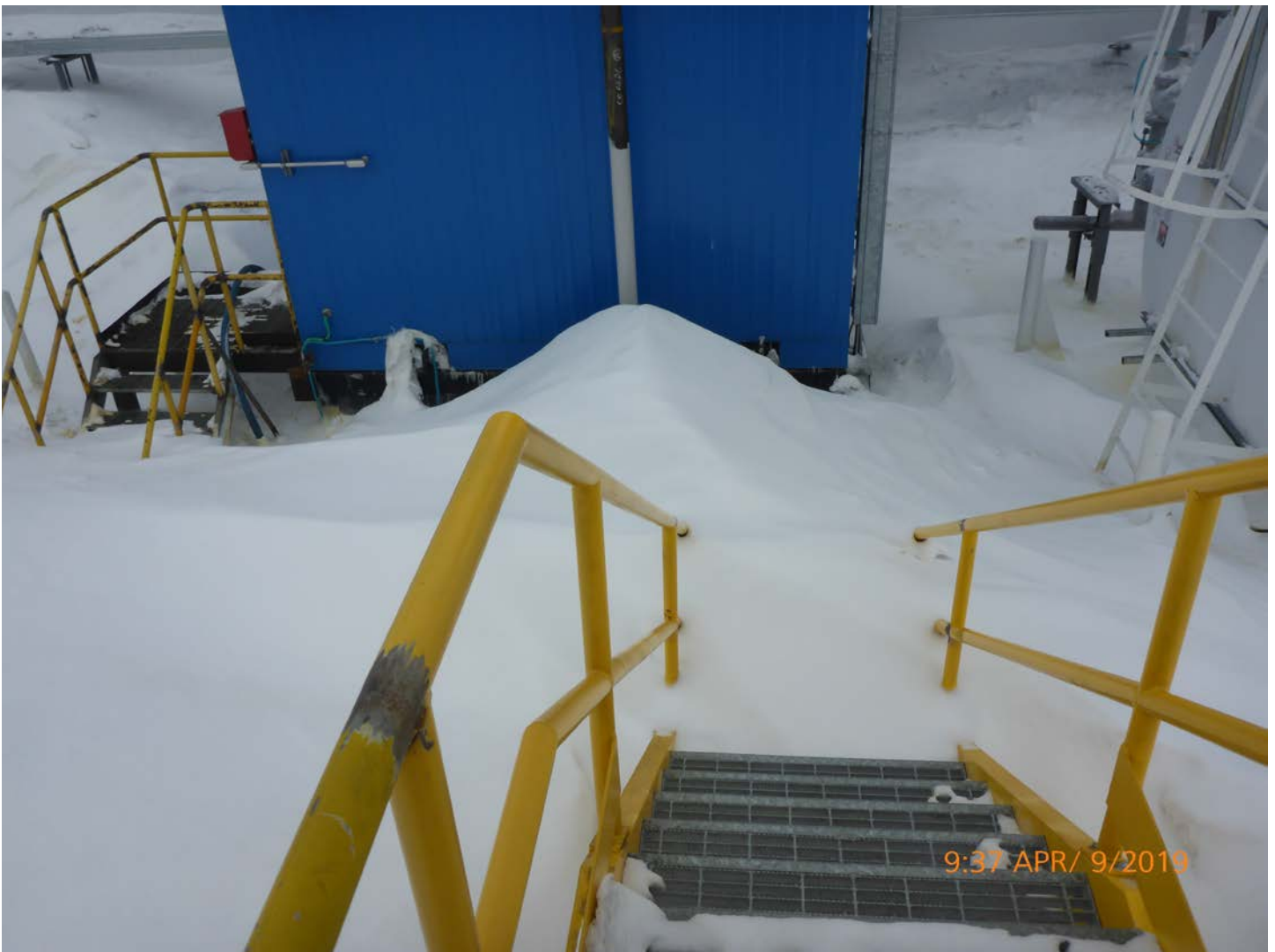
Photo 10 – Tank Farm Spill #2019127 – Access to the day tank in the sable fuel farm was snowed in, which made the tank difficult to inspect. The Inspector recommends better maintenance at the access points to the tank farm containment to facilitate inspections.
