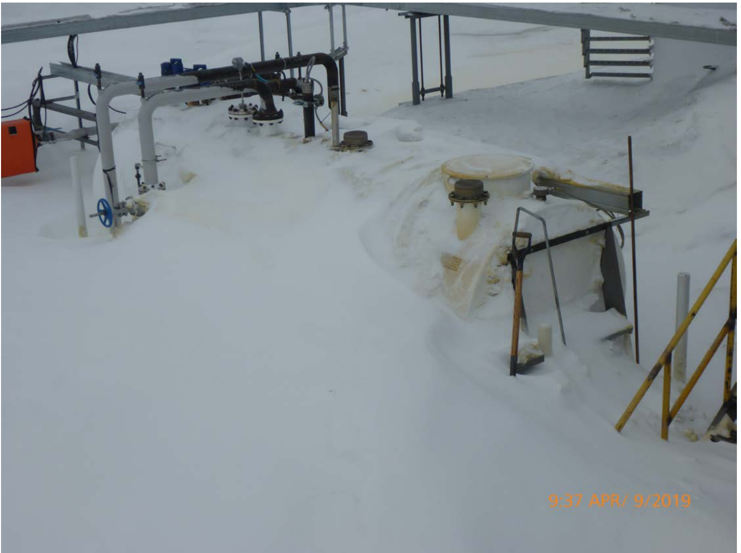
Photo 9 – Tank Farm Spill #2019127 – The 9000L generator day tank was overfilled when the automatic shutoff switch froze open.
