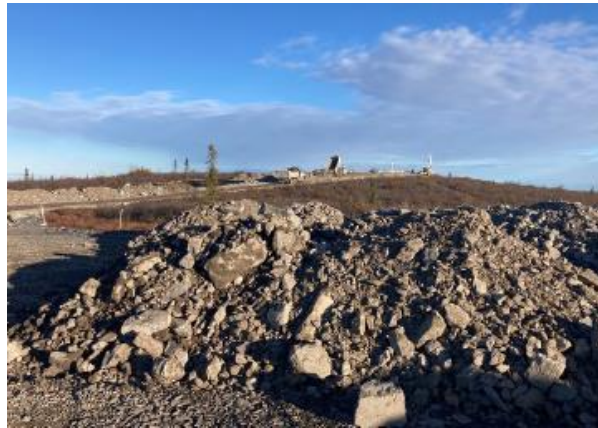
Dumping on Crane Pad
