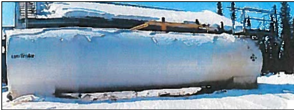
Figure 3 – Diesel fuel tank.
