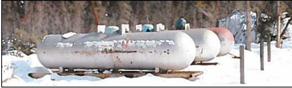
Figure 4 – Three 4,500 L propane fuel tanks
