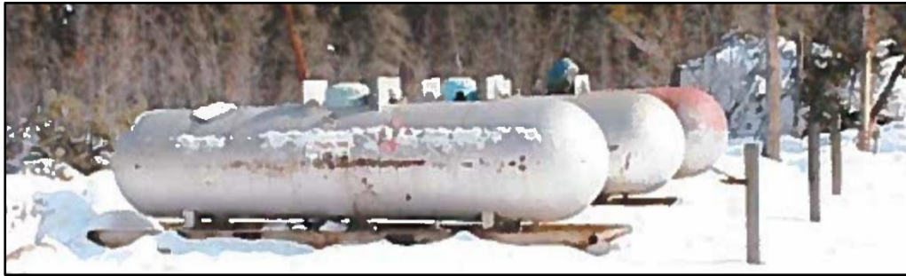
Figure 4 – Three 4,500 L propane fuel tanks
