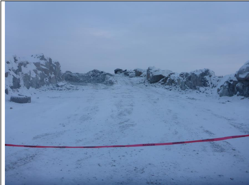
Photo #1: Overview of the blasting area located northwest of the C-Dry building
