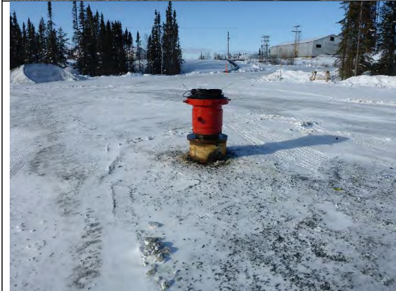
Photo #4: Akaitcho pump #1 overview.
