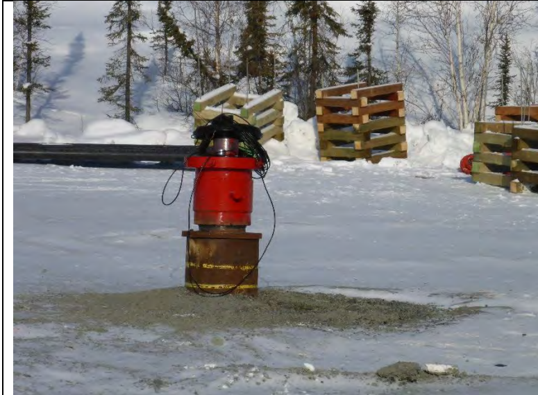
Photo #2: Akaitcho pump #2 overview
