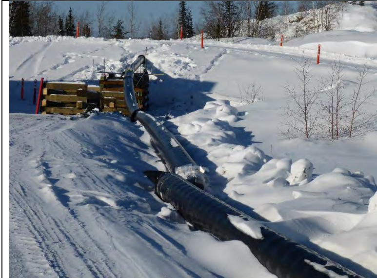
Photo #7: Piping installed that runs from the pumping area to the Northwest Pond.
