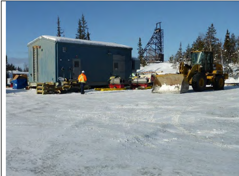
Photo #1: Overview of the pumping location.
