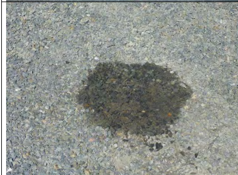
Photo #6: Multiple small hydrocarbon stains located around the Akaitcho pumping station.
