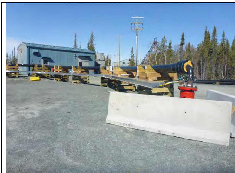
Photo #5: Overview of the Akaitcho pumping location.
