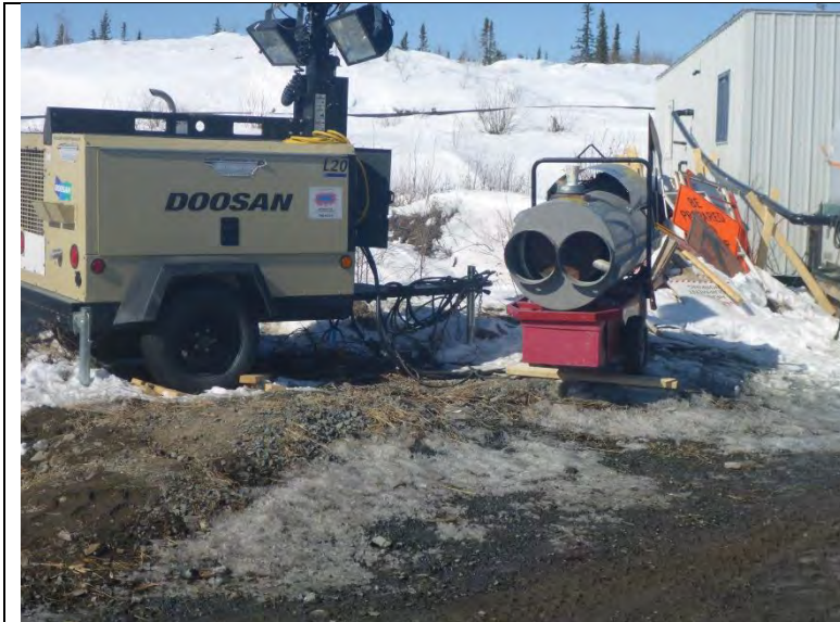
Photo #1: Overview of the camp setup near the drilling site. Note the lack of drip trays present under the equipment.
