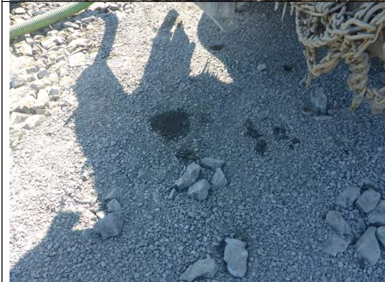
Photo #4: One of multiple small hydrocarbon leaks throughout the site.
