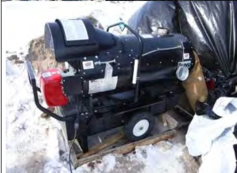
Photo #8: Photo 7 mitigation post inspection.
