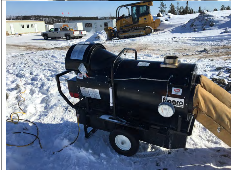
Photo #3: Frost Fighter at Alimak that does not have proper secondary containment.
