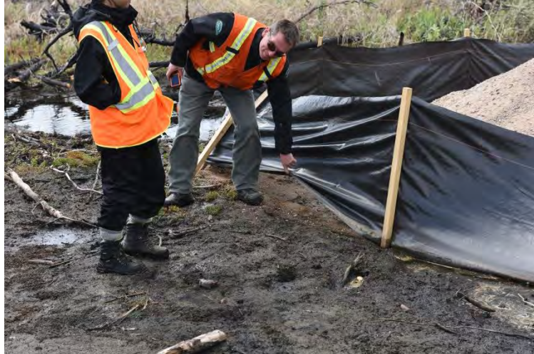
Photo #9: Silt fence at Joon Site. The silt fence was not properly tied into the ground.
