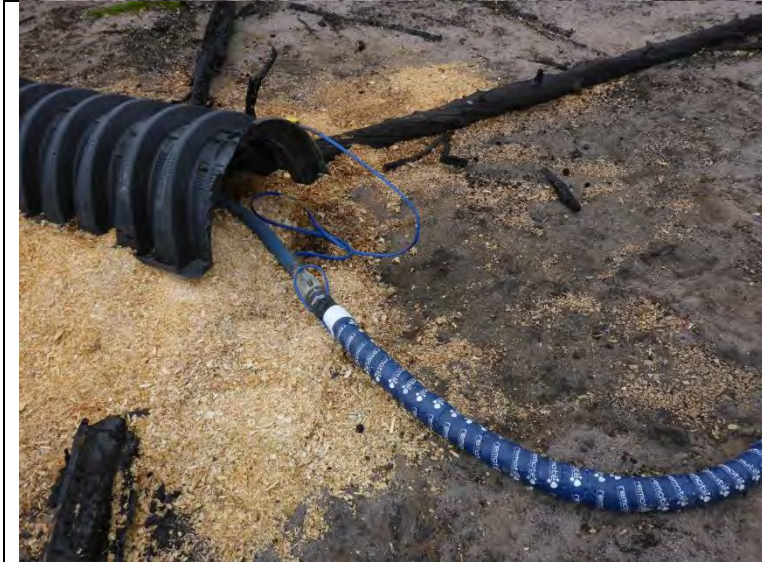
Photo #2: Close up of sewage discharge system. Note the electrical cord marking where sewage samples can be taken.
