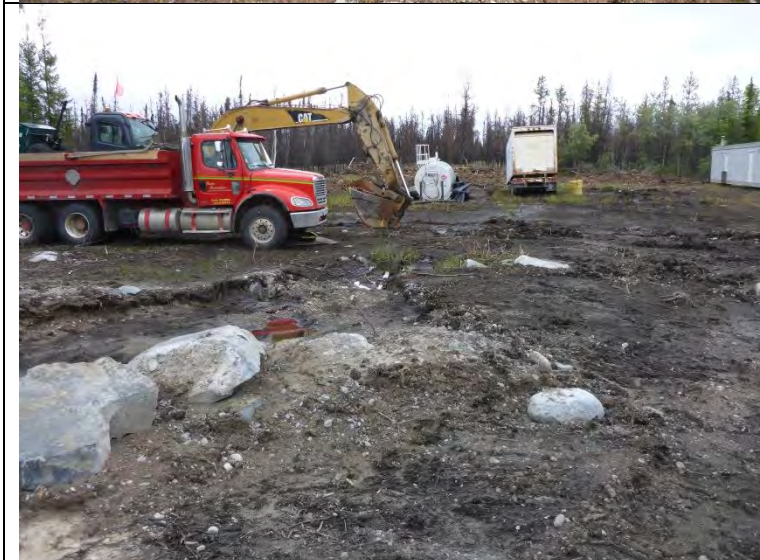
Photo #6: Beaulieu Site. Note that most of the water has been drained.
