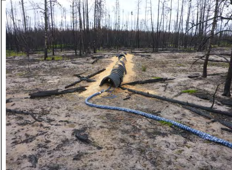
Photo #1: Set-up of sewage discharge system. The discharge pipe is covered and slowly discharges into the sawdust.
