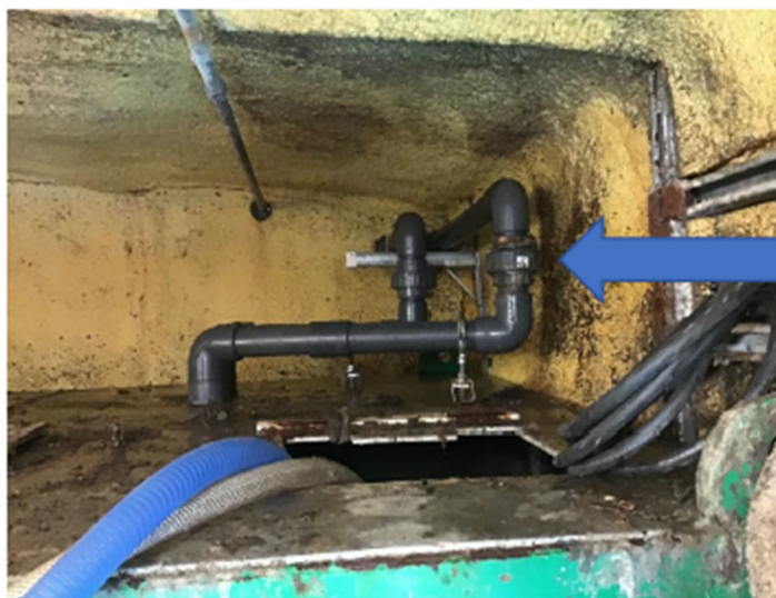
The cracked line located behind a tank in a difficult area to assess
