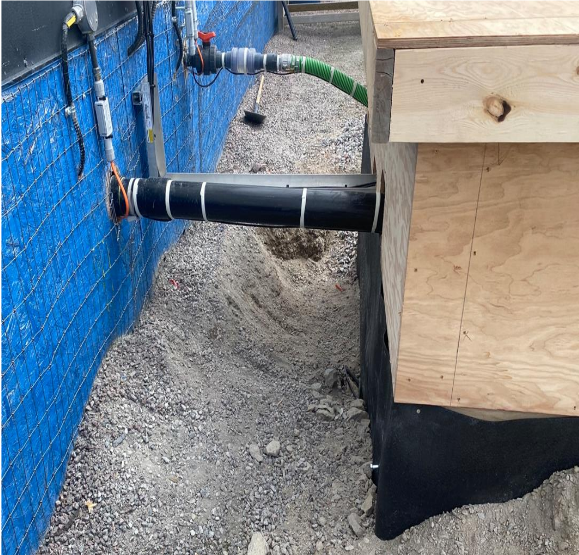
Figure 3. Verification of spill clean up, GNWT Spill #2024216
