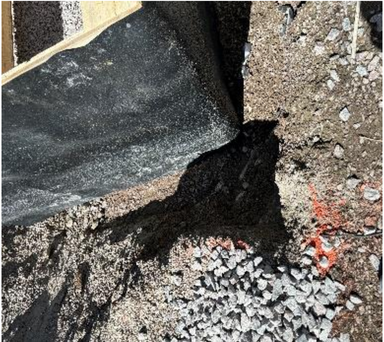
Figure 2. Spill at Dorm A11 Lift Station, GNWT Spill #2024216
