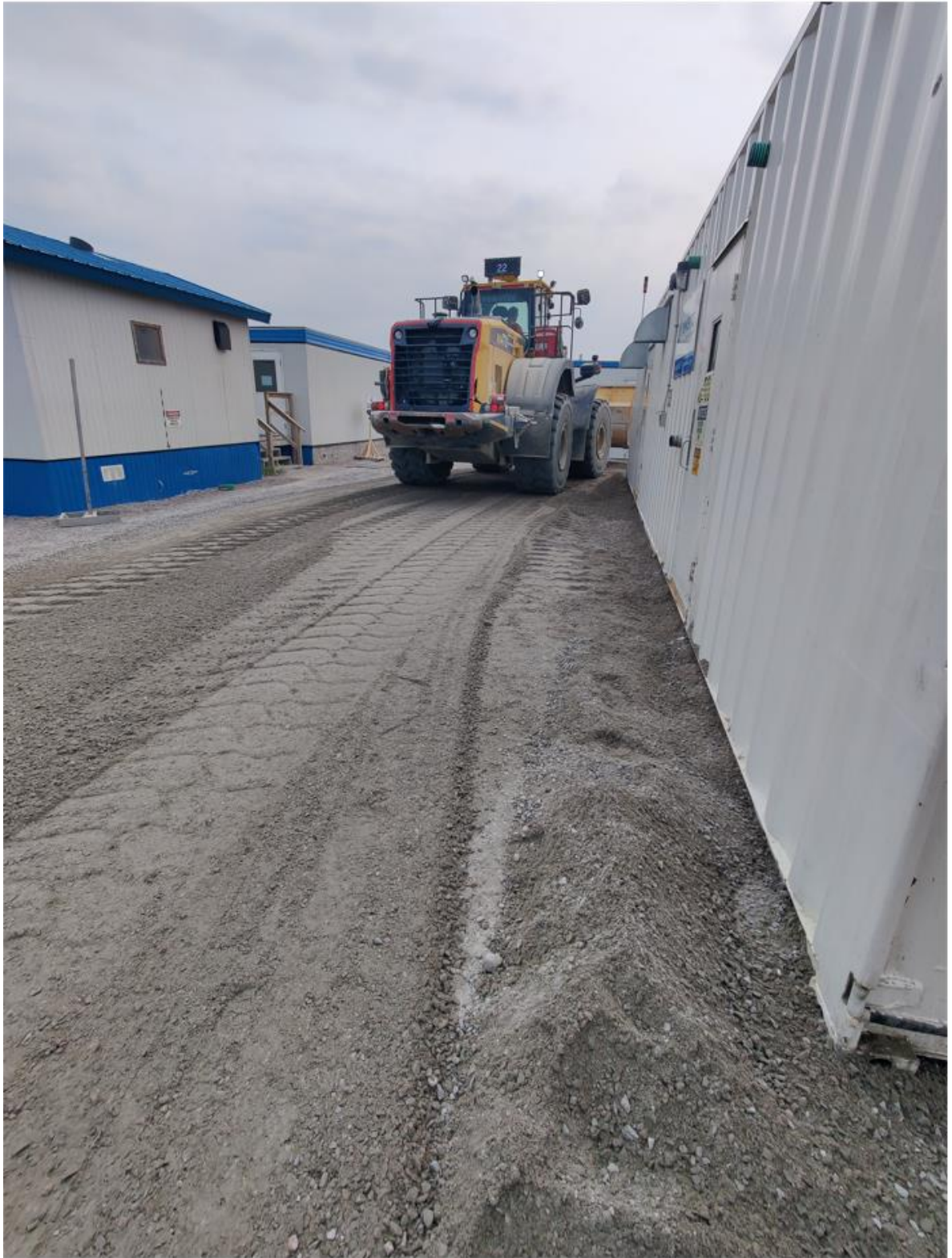
Figure 4. Photo of the affected area once remediated GNWT Spill #2021309
