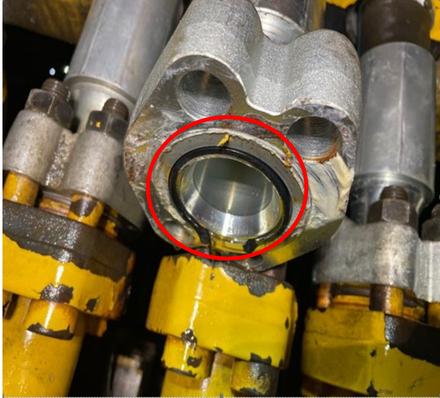
Figure 3. Failed O-ring Found upon Investigation of Failure Resulting in GWNT Spill #2021378
