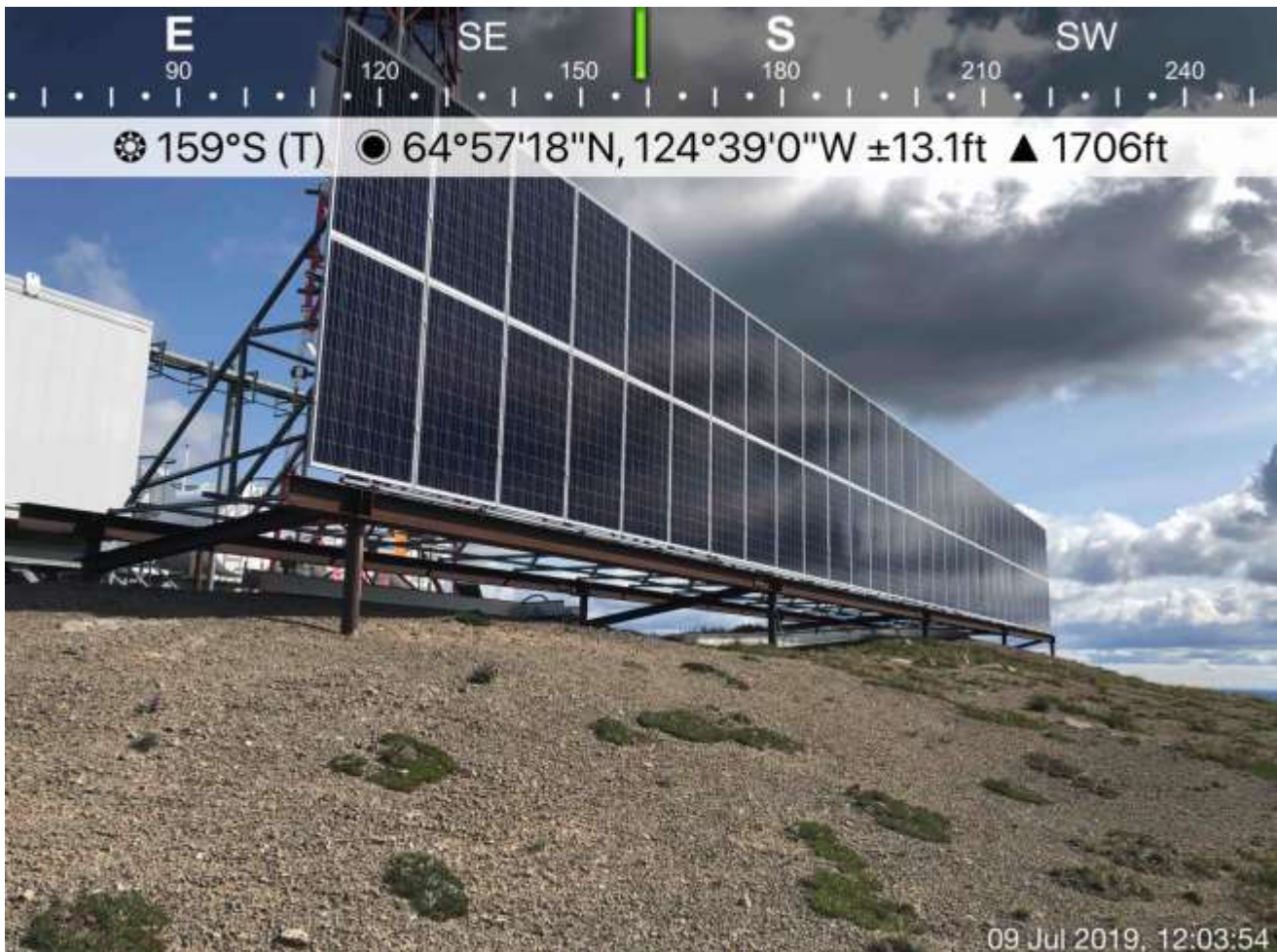
Larger solar panels
