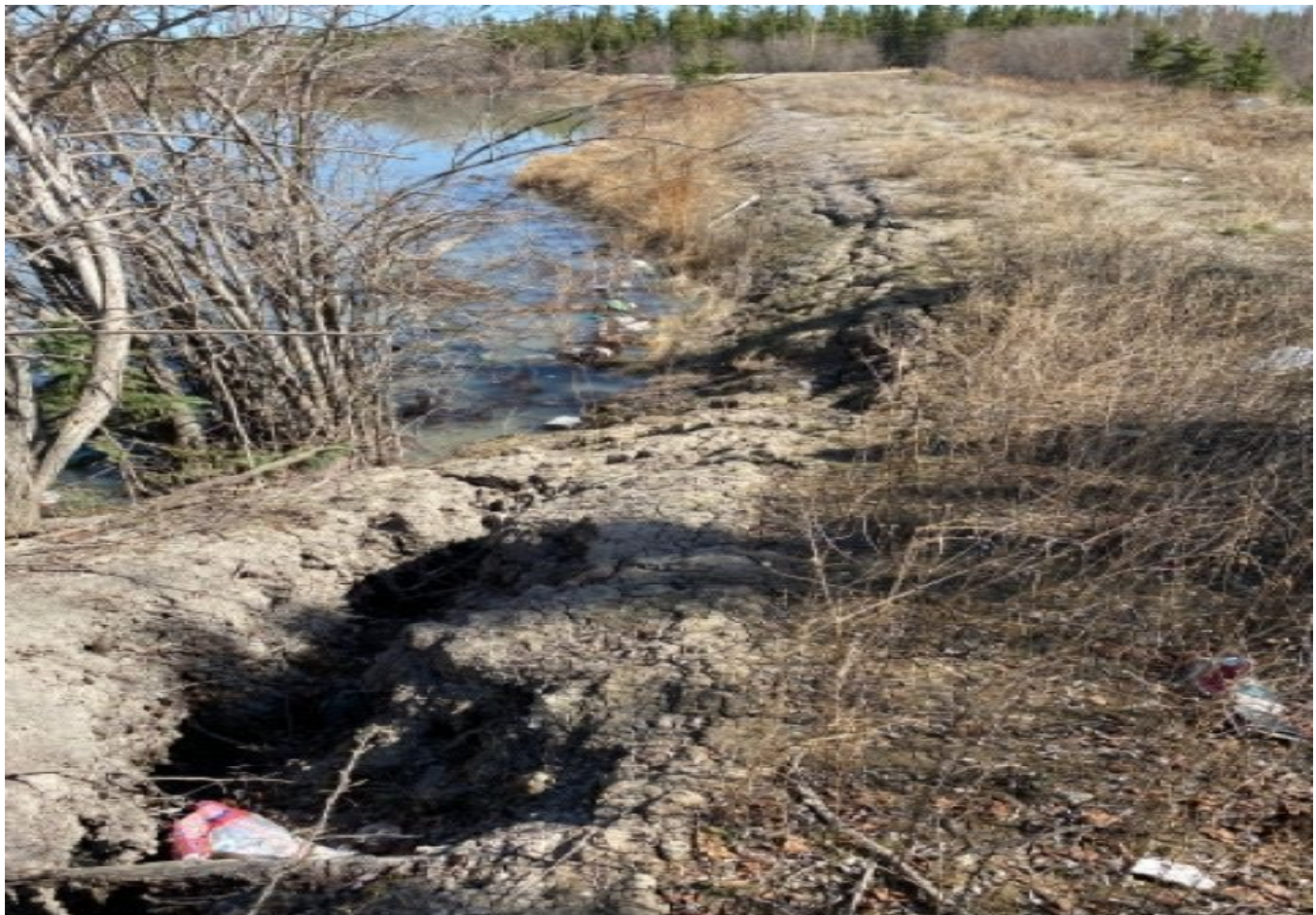
Photo 2 - Crack in berm of Cell 1 at Rae Sewage Lagoon
