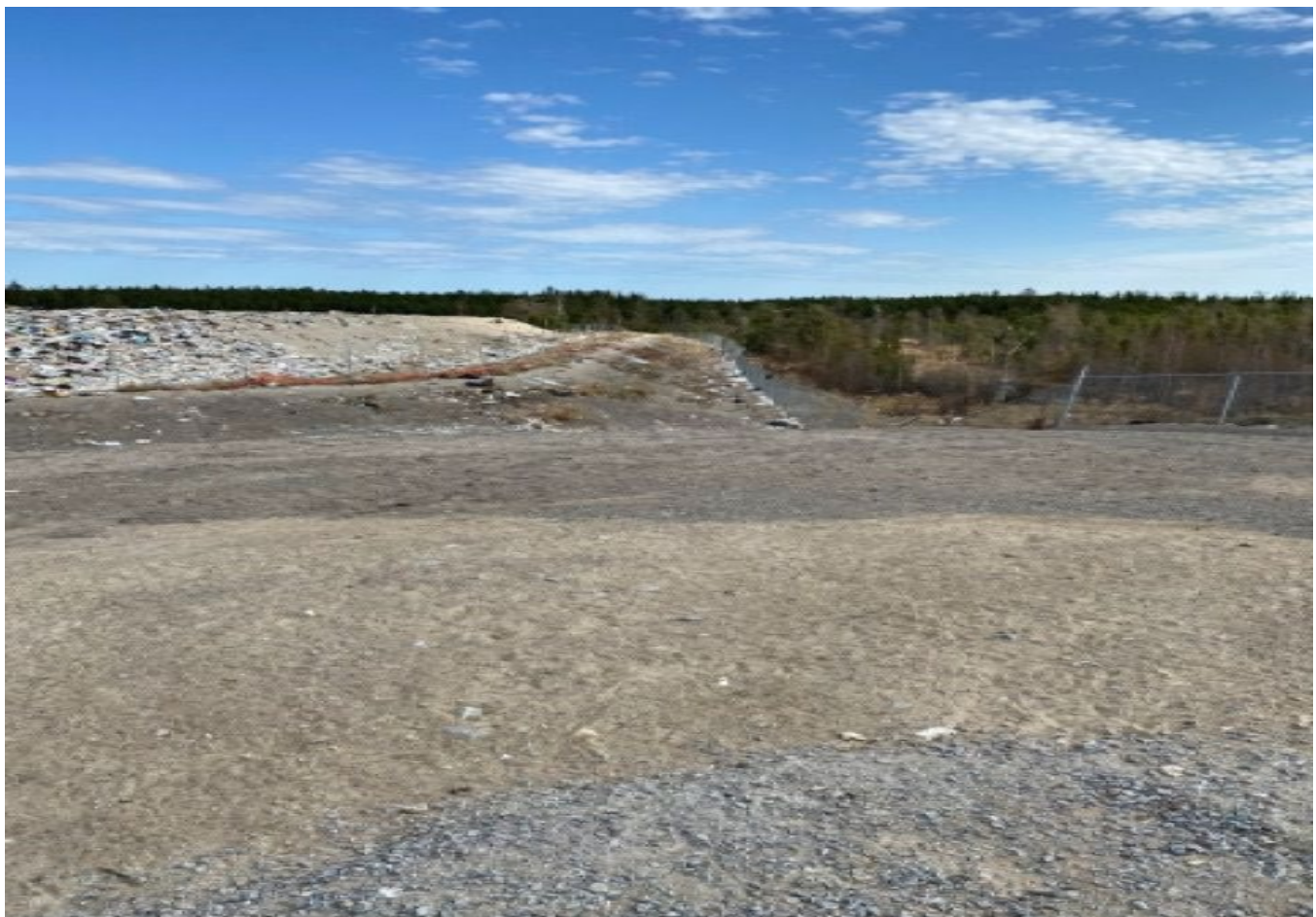
Photo 6 - Solid waste facility fencing requiring repair
