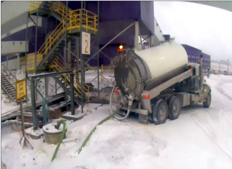
Figure 2 Sewage hose connected to lift station prior to spill.
