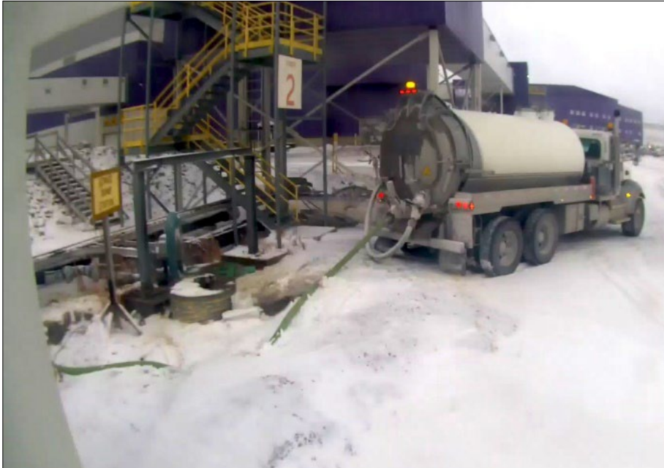
Figure 3 Disconnected hose at lift station and raw sewage spill.
