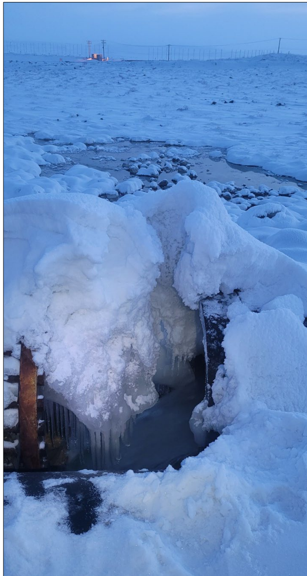
Figure 2. Spill 2023102 – Water flow at damaged dewatering pipeline in the North Inlet Containment Facility area.
