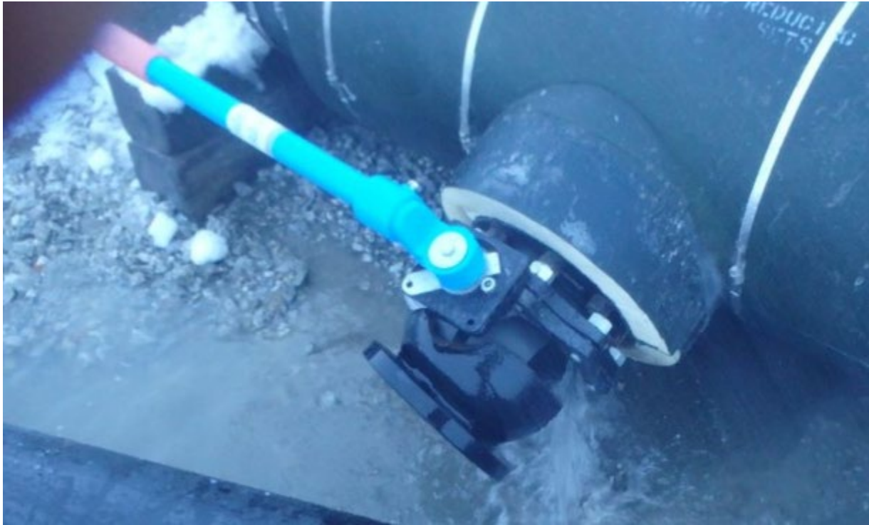
Figure 2 Broken valve during release
