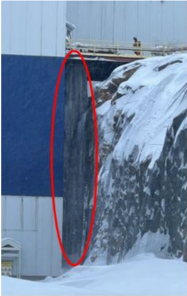
Figure 3 Ice buildup outside Process Plant.
