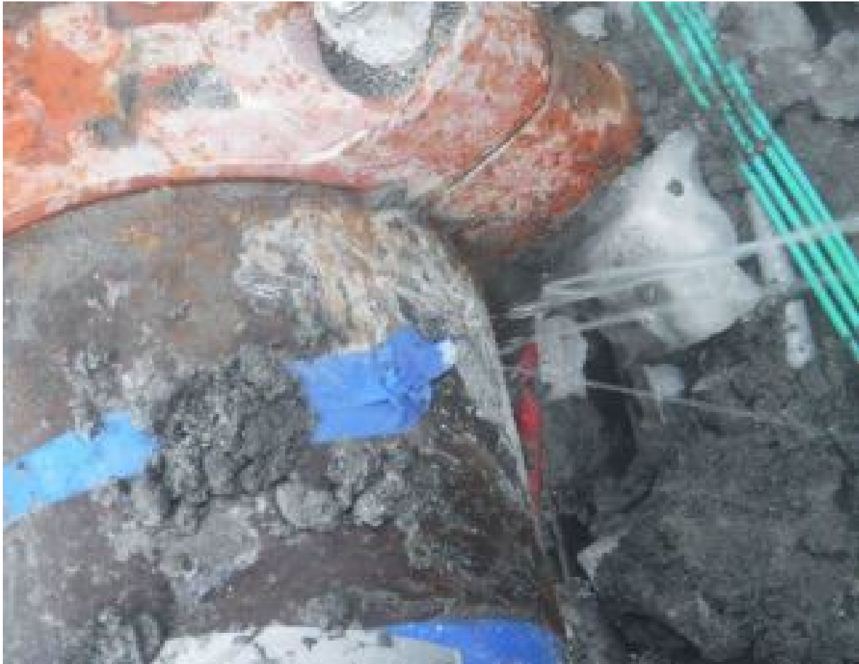
Figure 2 Leaking valve on PKMW line #311
