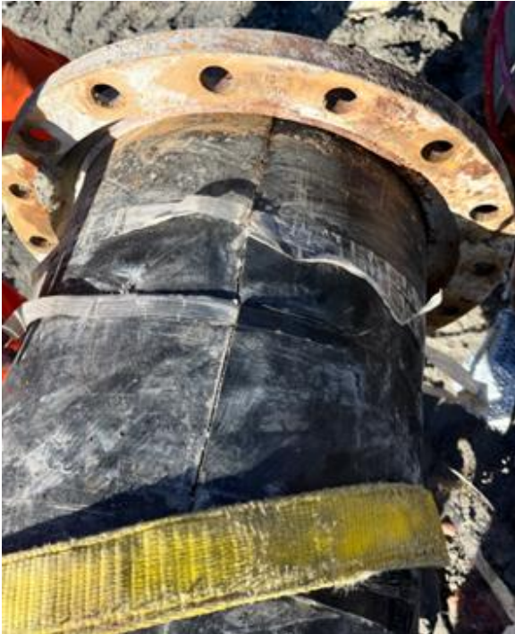
Figure 3: Crack in Process Plant Wet Well pipeline at flange
