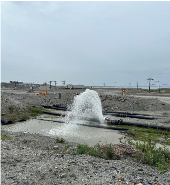
Figure 2: Extent of spill in front of Backfill Plant
