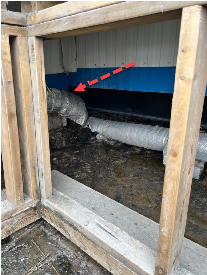
Figure 2: Location (red arrow) and extent of spill beneath E-Wing dormitory
