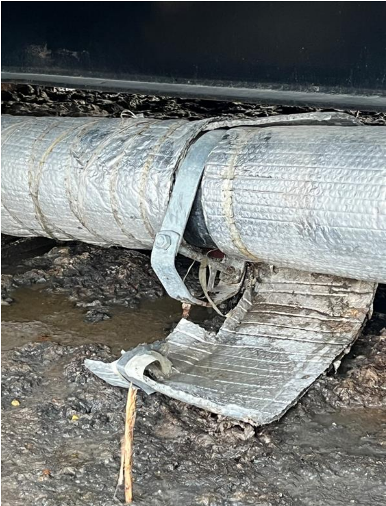
Figure 3: Failed pipe hangar
