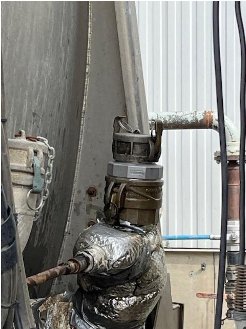
Figure 4: Tank trailer fill valve closed
