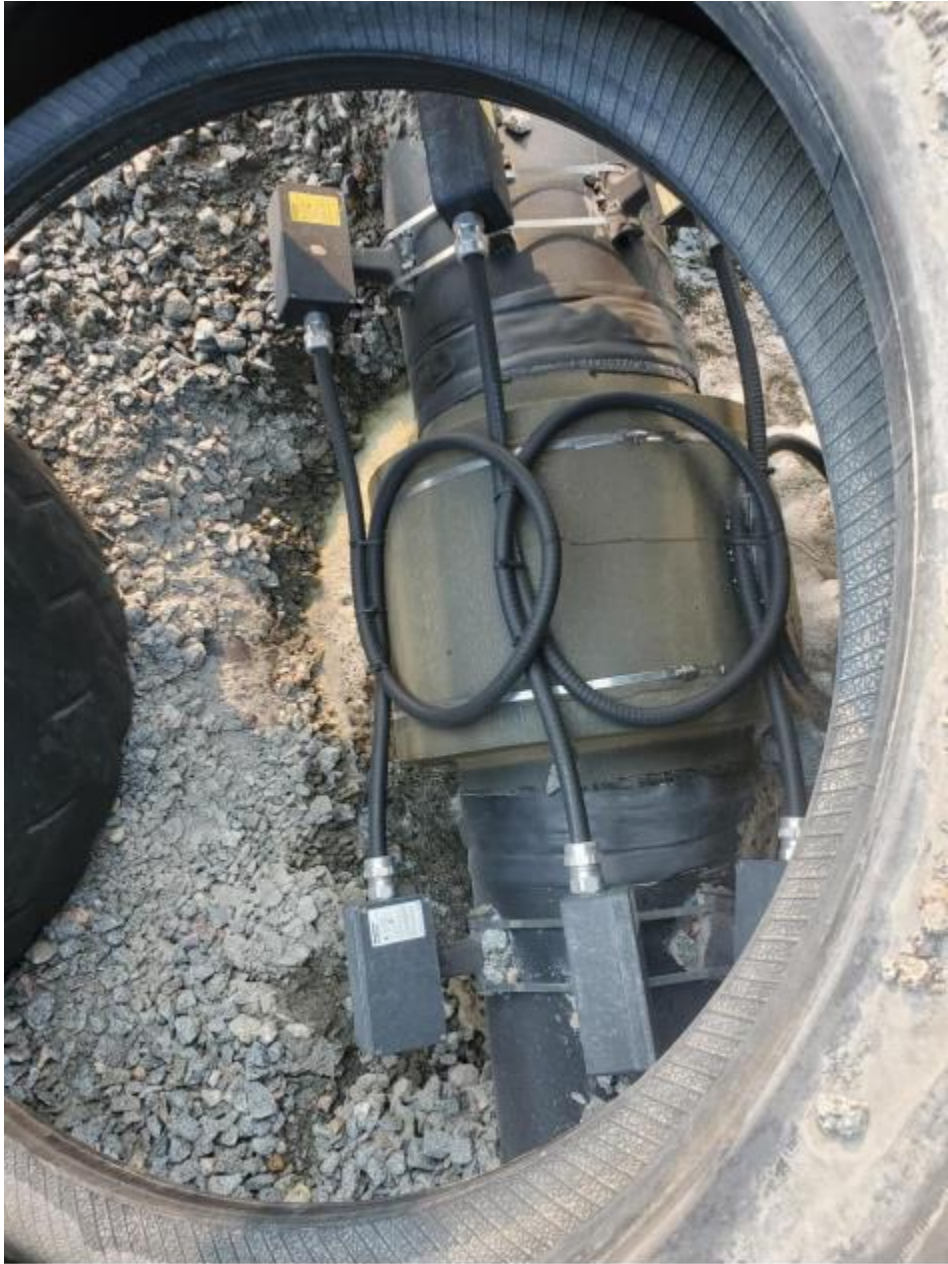
Figure 3: Location of spill after pipeline flow was turned off.
