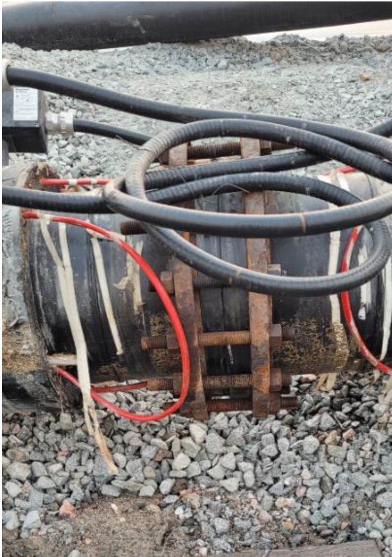
Figure 4: Failed gasket removed and joint bolted.
