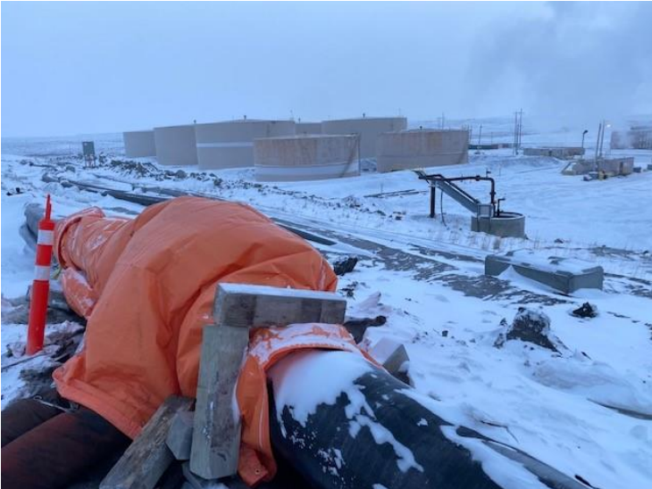
Photo 1: Facing E Spill 2022547 immediately after spill occurrence placed a cover over the damaged area of Koala tailings line.
