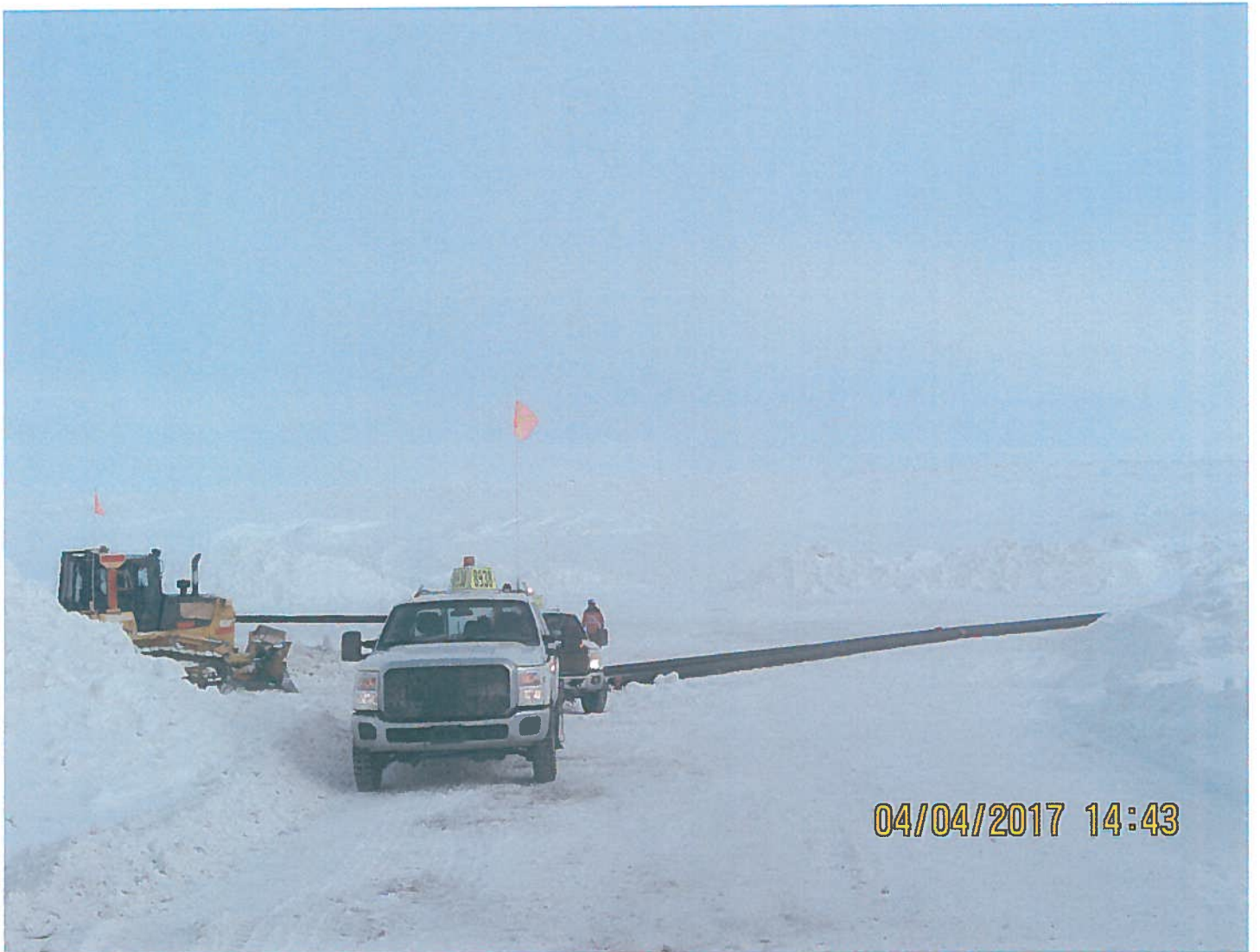
Photo 7: Sable Lake Dewatering Line - A 10" HDPE temporary dewatering line was being pieced together on Sable Lake during this inspection. The dewatering line will be placed in frozen conditions running from Sable lake to Ulu Lake
