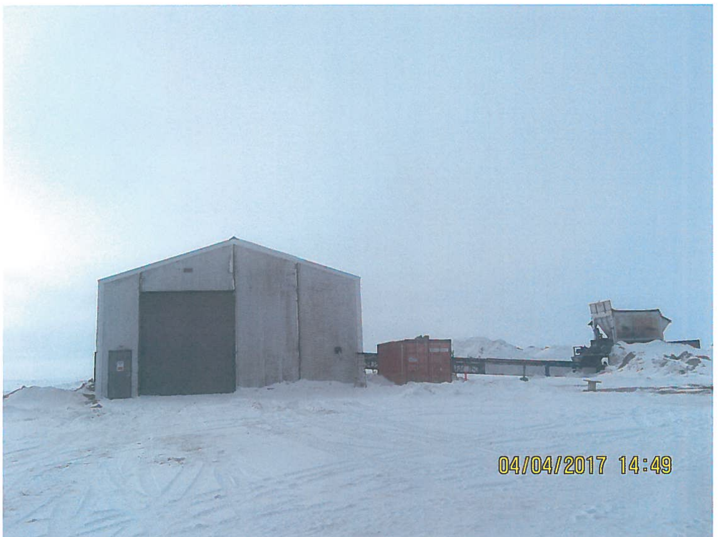
Photo 3: Frozen Core Plant - The Frozen Core Plant will be decommissioned in the near future. All components for this facility will be removed and stored at the Nuna Zone 12 laydown area at main camp.
