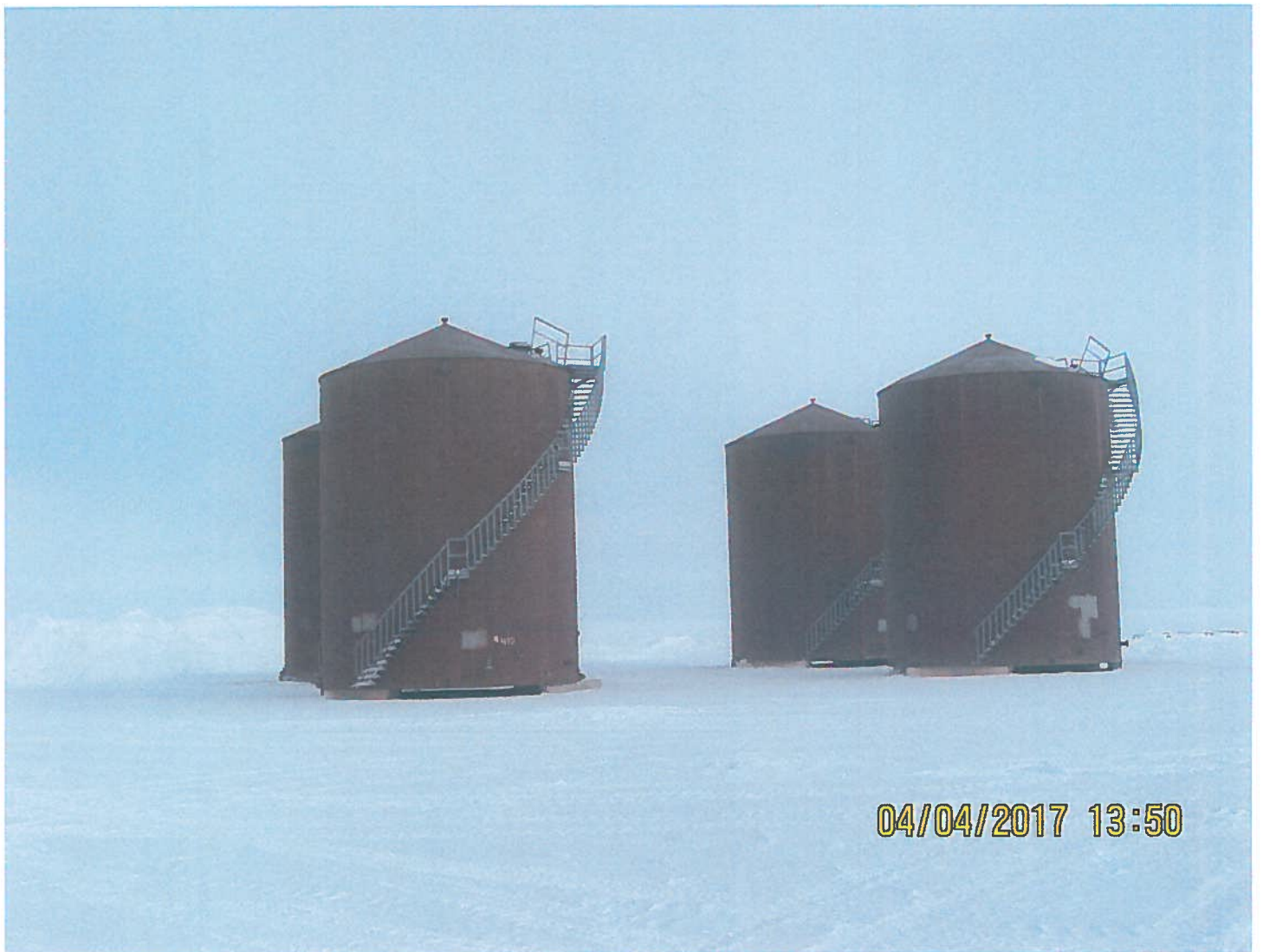
Photo 1: Sable Office Complex Laydown Area - Four - 500,000 Litre fuel tanks will be placed in an engineered berm at the Sable Office Complex Laydown Area.
