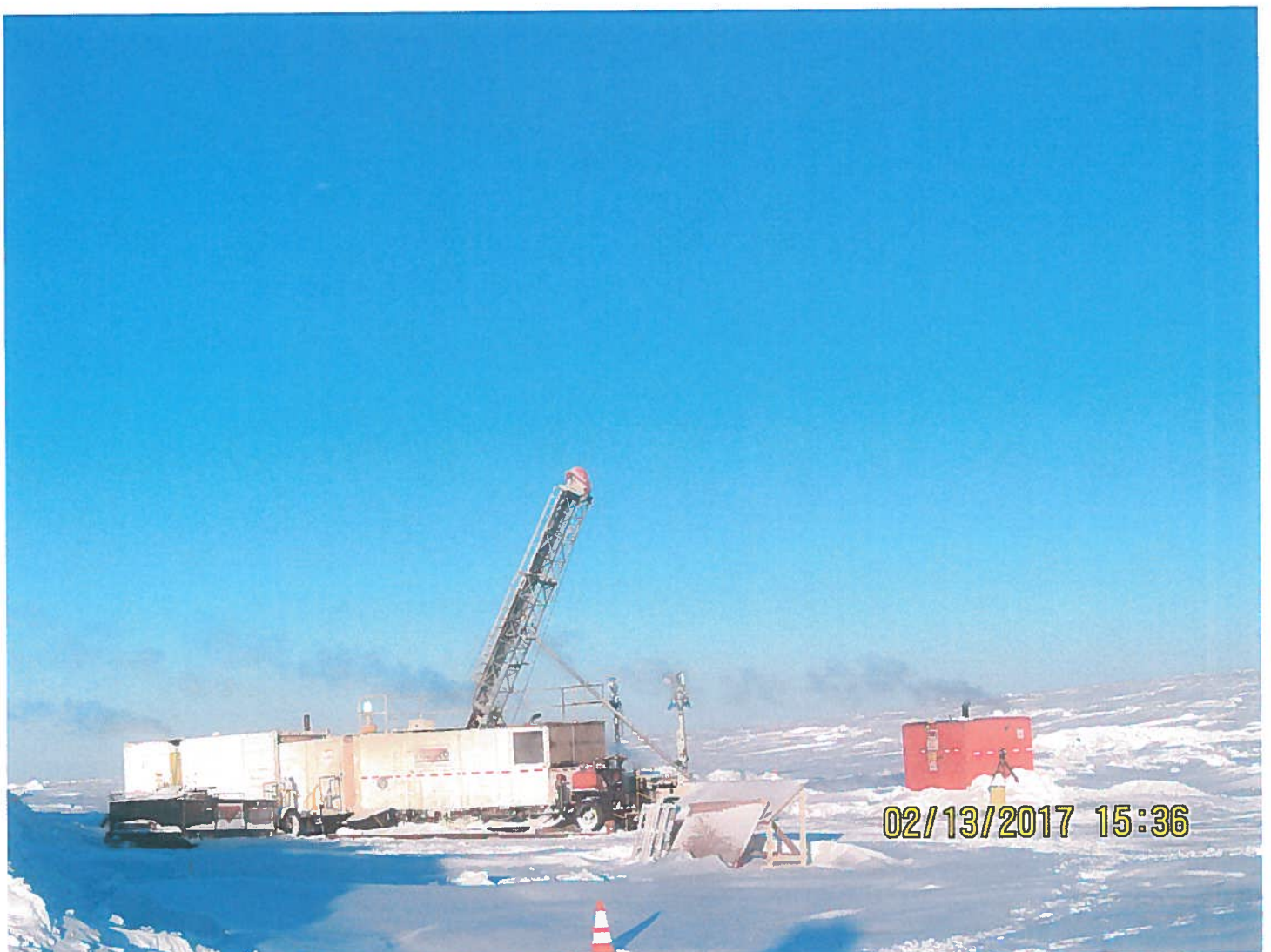
Photo 8: Sable Development/Sable Lake- Foraco Drill Shack and generator on Sable Lake. Geotechnical drilling will be completed in the last week of February.
