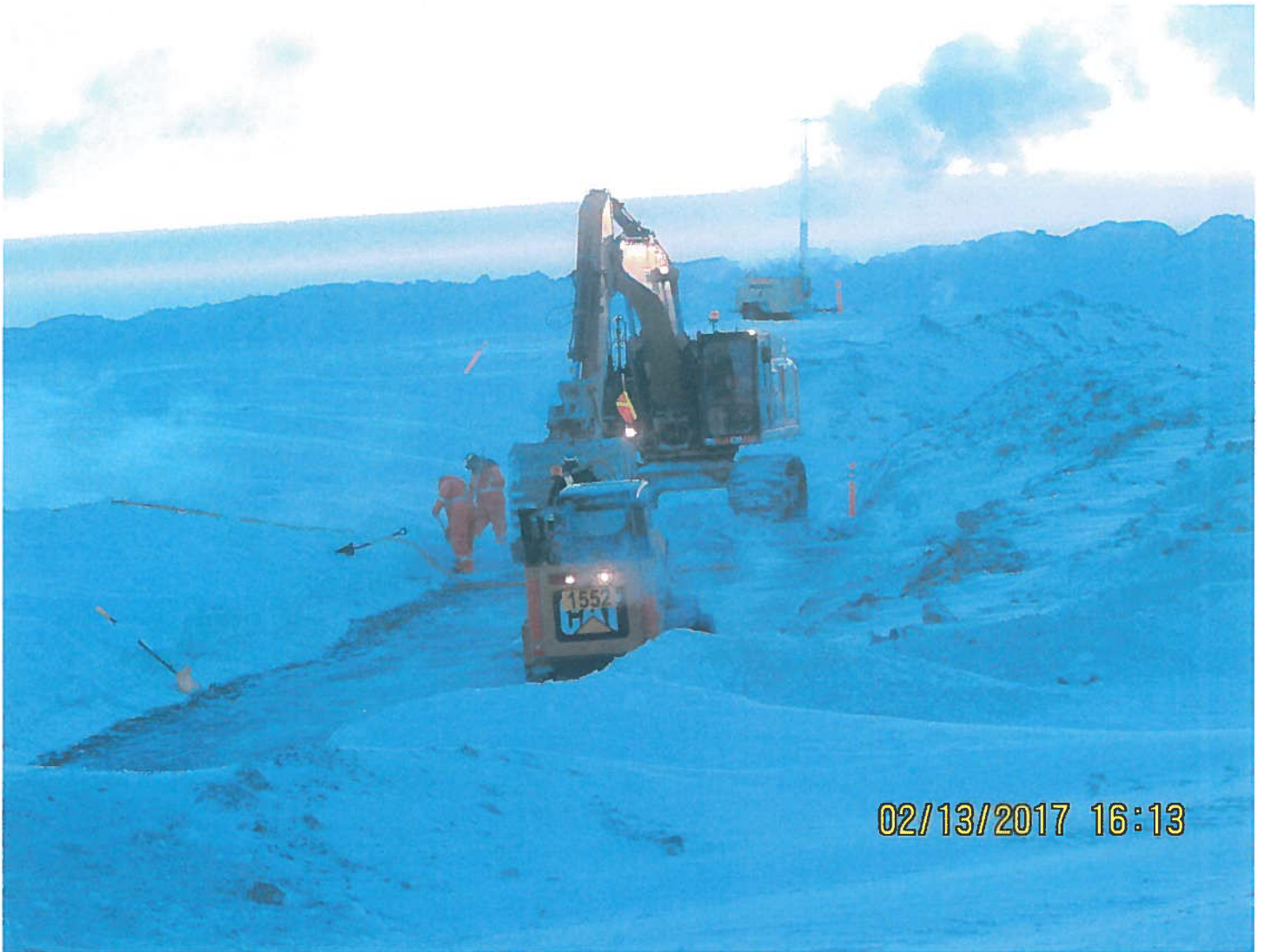
Photo 3: Sable Development/Frozen Core Dam- Nuna staff preparing the frozen core dam surface for the next layer of slurry. The surface needs to be free of snow to ensure there is a solid bond between the slurry layers.
